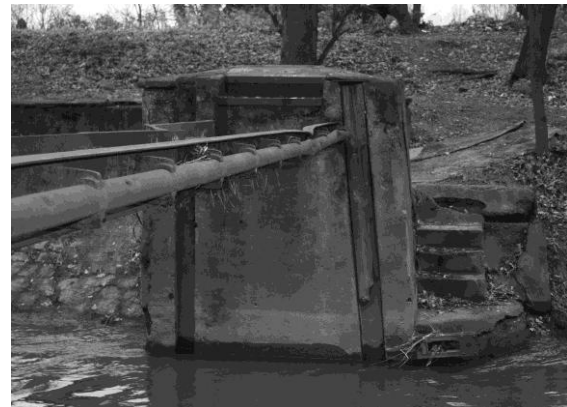
Figure 5. The fortress weir XI ( Nadelwehr - St. W. XI ) in a state of major disrepair, 2012 (Source: photo by the author, 2012)
