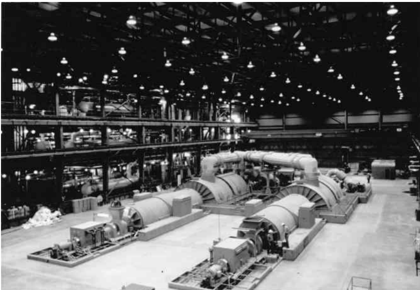
FIGURE 1.4 An installed 1300MW cross-compound turbine generator.
