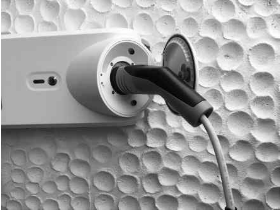
FIGURE 11.8 Home charging unit in Ireland
