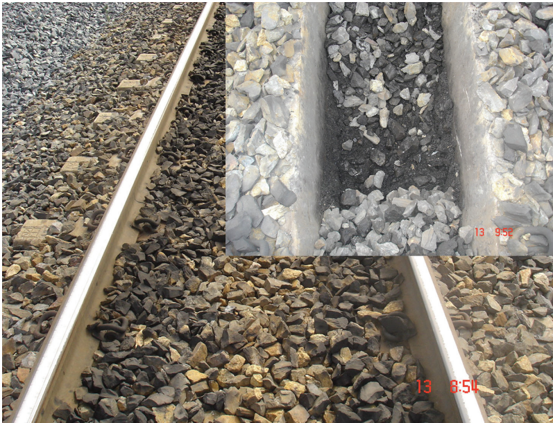
Figure C8 Migration of coal fines towards bottom of the ballast bed due to vibration and rainwater infiltration, leaving the surface ballast relatively clean – a site near Rockhampton.
