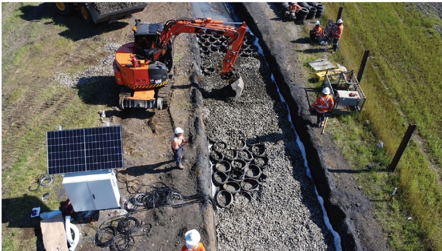
Figure E1 Placing rubber tyre cells in fully instrumented rail track at Chullora Technology Precinct, New South Wales.
