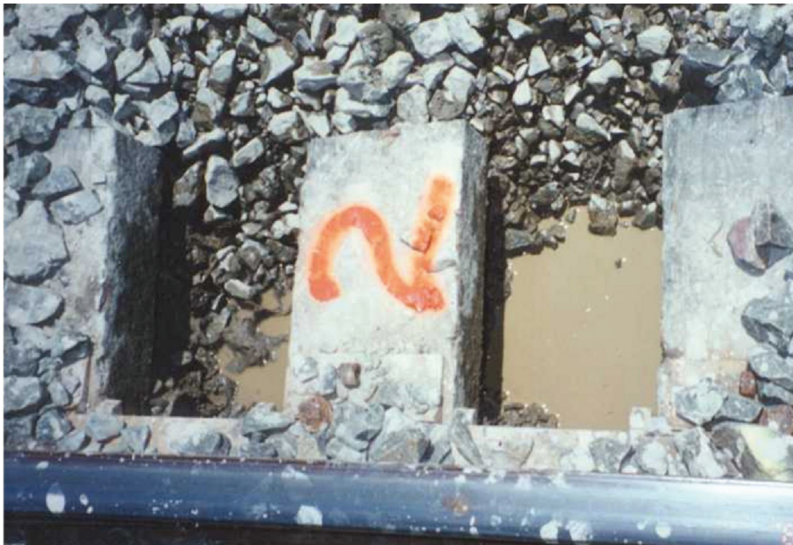
Figure 1.6 Ponding water in the load-bearing ballast along a Sydney metropolitan line in Australia.
