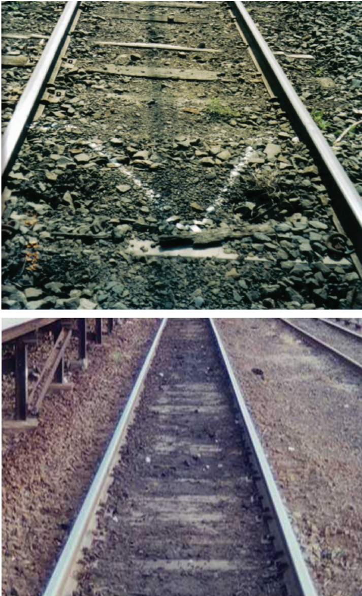
Figure 1.1 Degradation and fouling of ballast in track in New South Wales Australia.
