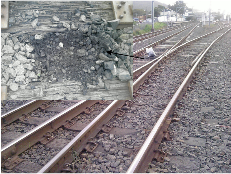
Figure C10 Pulverisation of ballast plus coal fouling observed near a v-crossing close to Thirroul, New South Wales.
