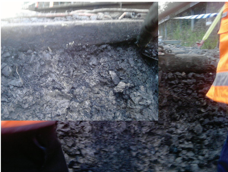
Figure C9 Coal and clay sediments fouling the ballast beneath the sleeper at a site in Thirroul, south of Sydney, observed during track maintenance.
