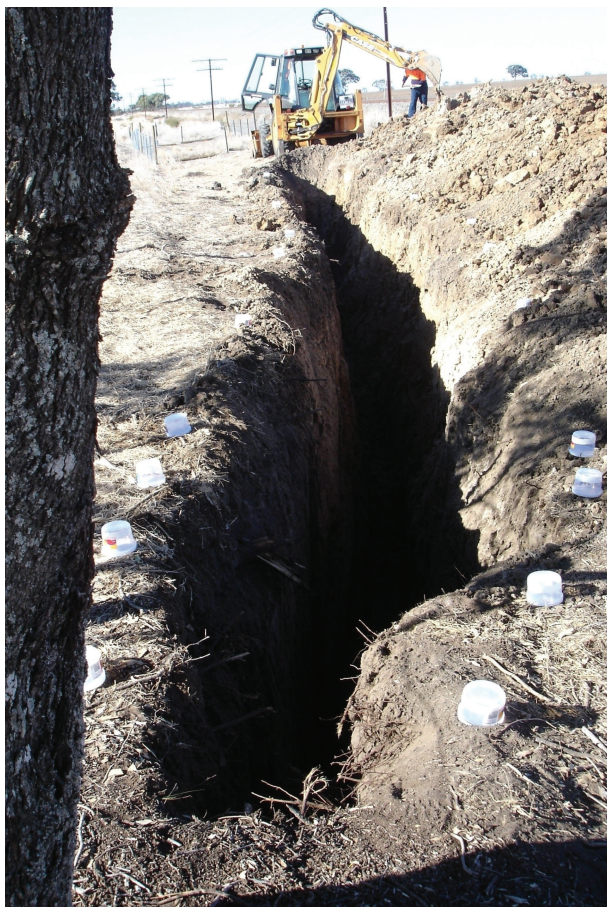
Figure 16.3 Trench excavation to examine the root density distribution of a native tree (Miram, VIC, Australia).
