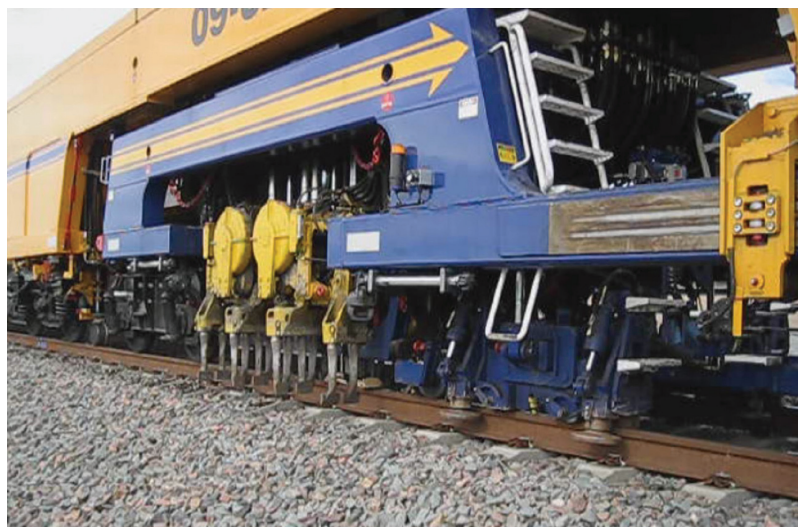
Figure 14.2 A closer view of the tamping machine showing tamping tines and lifting rollers.
