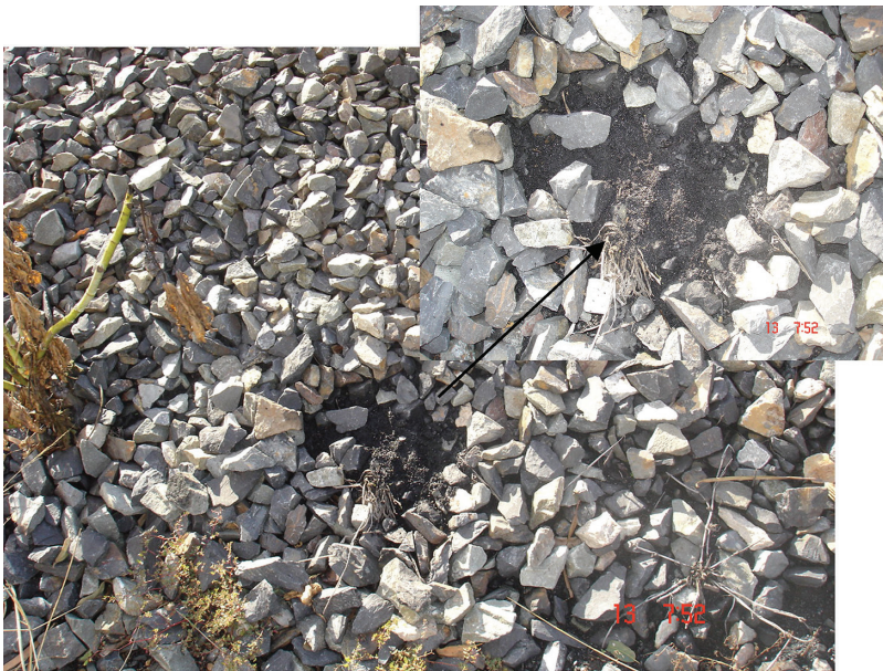
Figure C7 Intrusion of coal fines into the shoulder ballast in a track near Rockhampton, Queensland.
