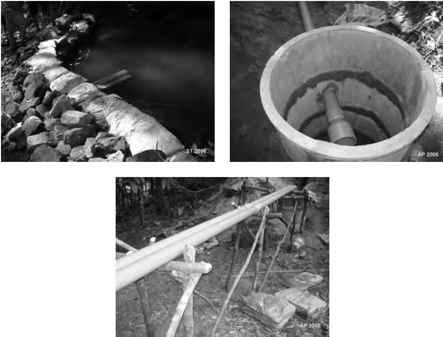
Figure 2.6 Photographs of the weir and intake (upper left), the settling tank (upper right) and the canal as installed in HKT.
