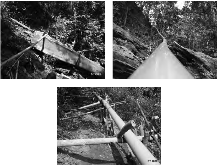
Figure 2.7 Photos of penstock as installed in HKT.
