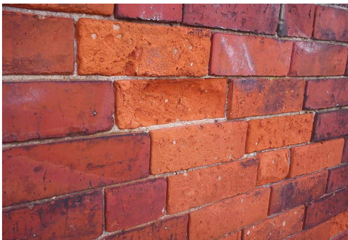
Fig. 267 Perished and spalled brickwork.
