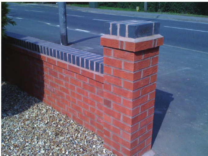
Fig. 236 Attached pier terminated higher than the wall.
