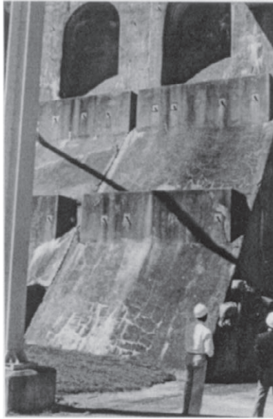
Figure 6.3 Cracking caused by alkali–silica reaction.
