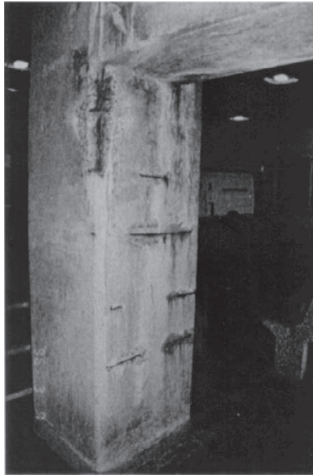
Figure 6.2 Inadequate cover of steel reinforcement.
