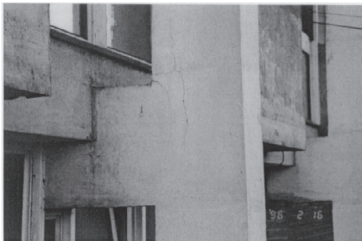
Figure 6.1 Structural cracks at a column beam connection.
