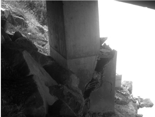
FIGURE 1.14 Column shear failure. (From Chile Earthquake, February 27, 2010.)
