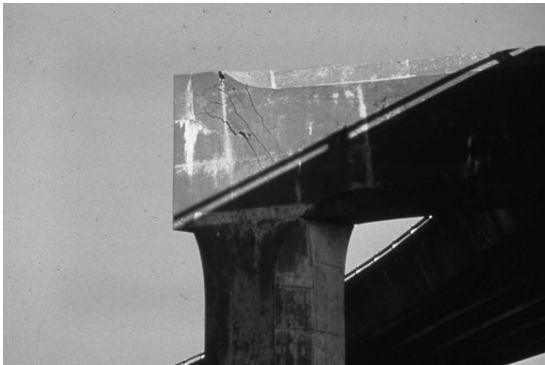
FIGURE 1.15 Cracking of beam-column connection. (With permission from Caltrans.)
