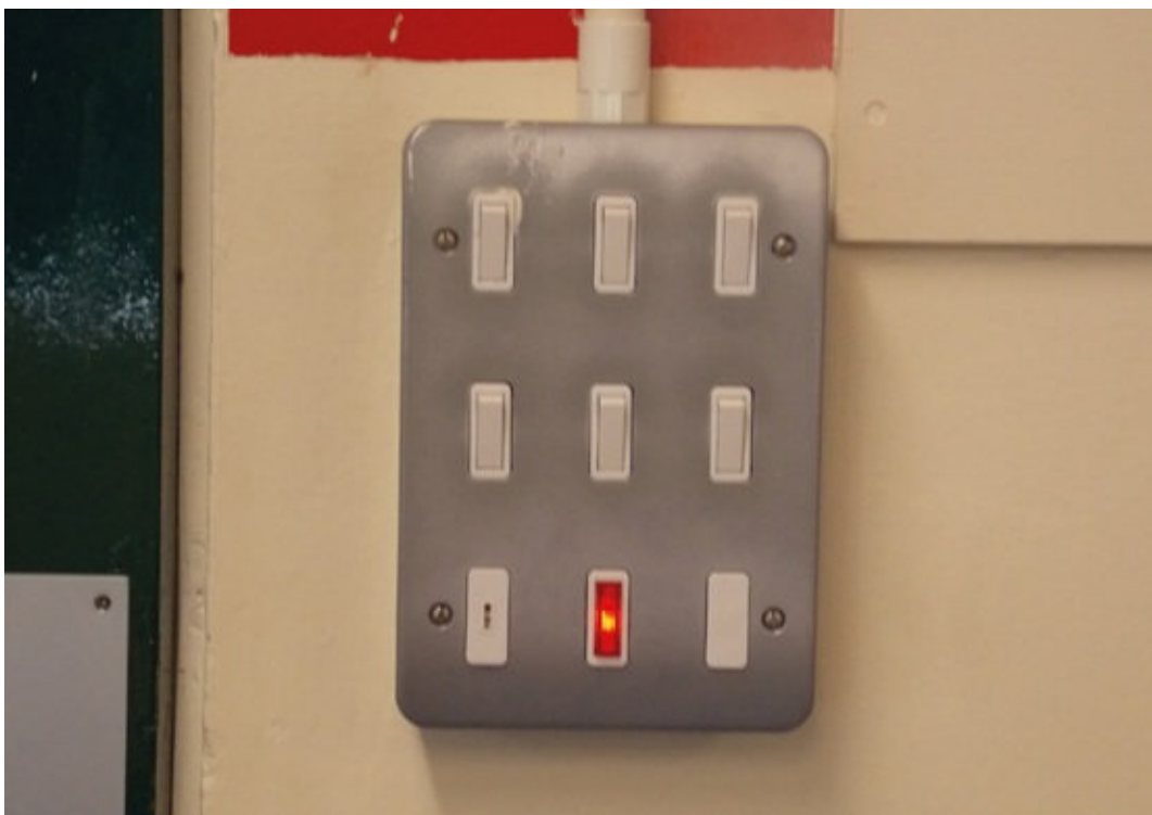
Figure 4.43 All parts of an Installation that are conductive (metallic) are known as exposed conductive parts and have to be earthed
