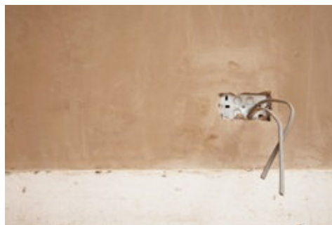
Figure 5.6 Various trades have to work together, such as an electrician and a plasterer
