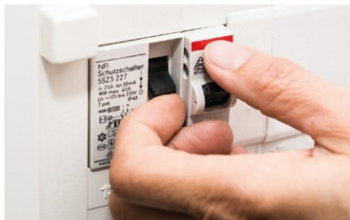
Figure 4.16 An RCD protects people, by isolating the circuit, if electrical current is not returned through the neutral conductor and flows to earth instead
