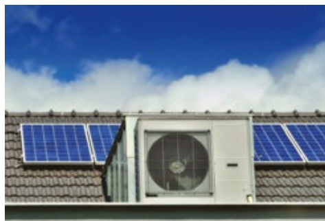
Figure 3.8 Solar panels installed in the northern hemisphere should be south facing
