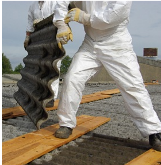
Figure 1.15 Asbestos must be removed by licensed and specialist contractors
