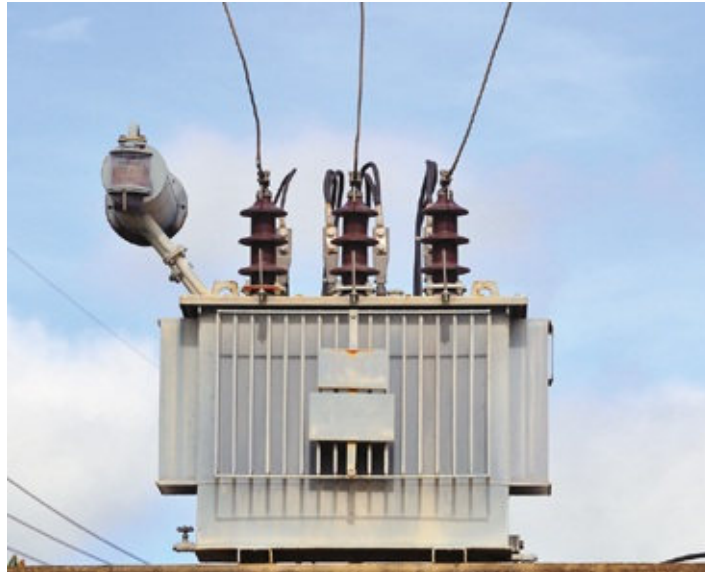
Figure 2.19 Transformers are used in the transmission and distribution of electricity
