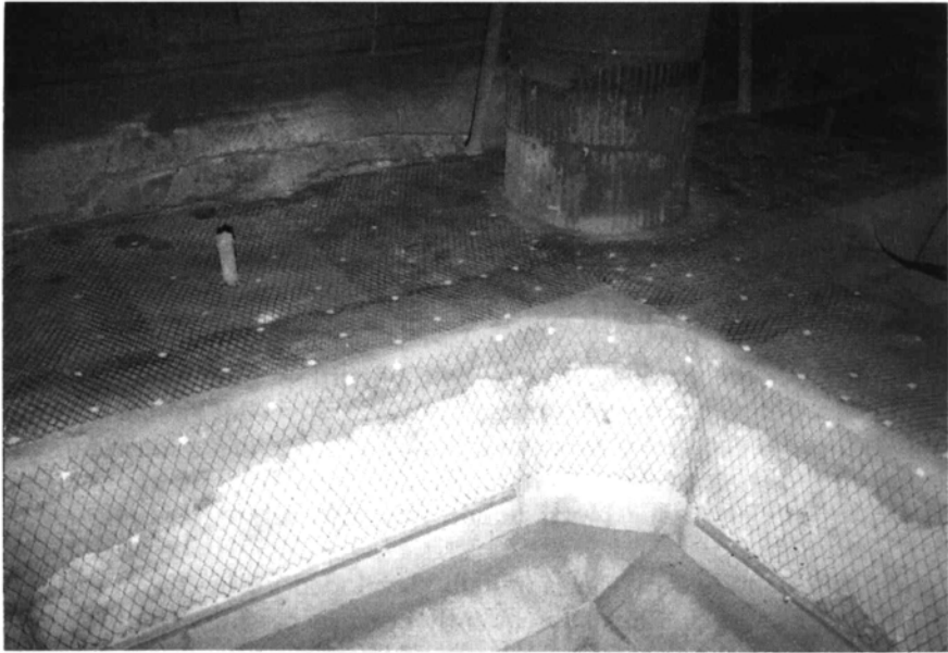
Fig. 7.1 Kwai Chung Jetty, Kowloon, Hong Kong. A double layer of anode mesh can be seen fastened to the concrete surface to provide a locally increased CP current. This increased current requirement is due to the greater embedded steel surface of the steel piles.
