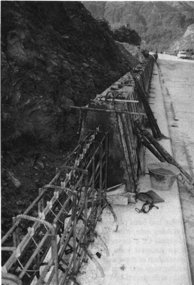
Fig. 7.5 Further CP application to the Turin-Frejus motorway bridges. This illustration shows a section of reinforcement cage complete with attached anode in front of a recently cast cathodically protected parapet.
