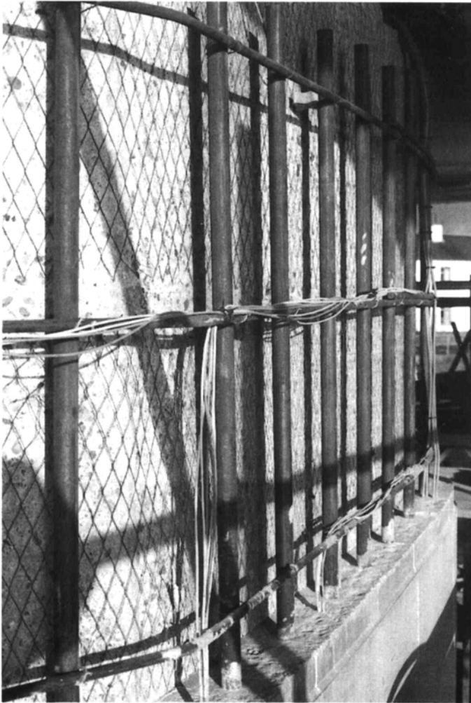
Fig. 7.2 Tay Bridge, Scotland. The base of a bridge pier which is being strengthened and provided with CP.
