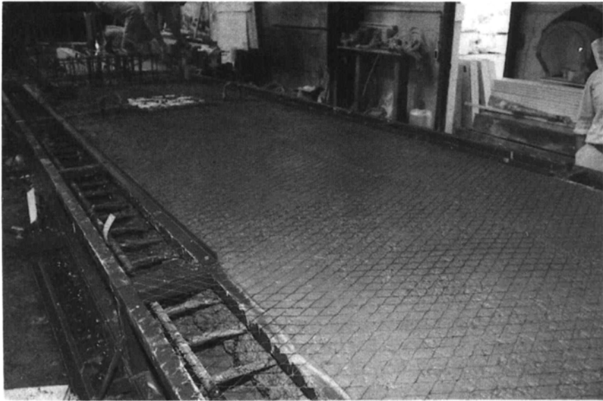
Fig. 7.3 A mixed metal oxide CP anode being cast into a newly constructed precast reinforced concrete element. These elements were used to form the pre-cast deck of a road bridge at Hauteville-sur-Fier, France.
