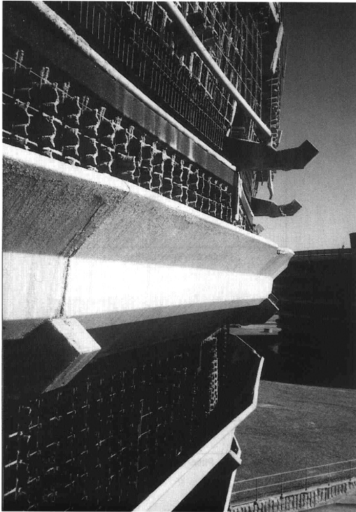
Fig. 1.5 Uncoated steel showing uniform corrosion in an exposed coastal environment.
