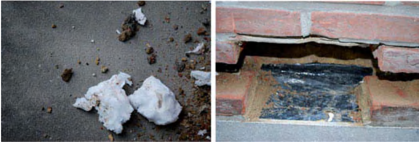
Figure 10.30. Post-fill with UF-foam (left), cavity tray with too low back flange as it looked after removing all mortar drops (right).
