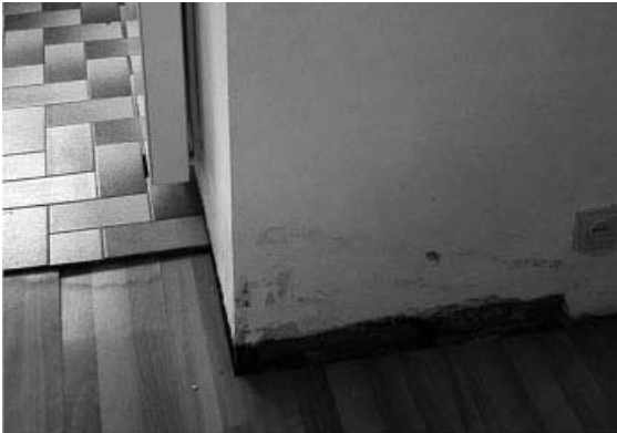
Figure 7.6. Floor in contact with bottom-wet partition wall.
