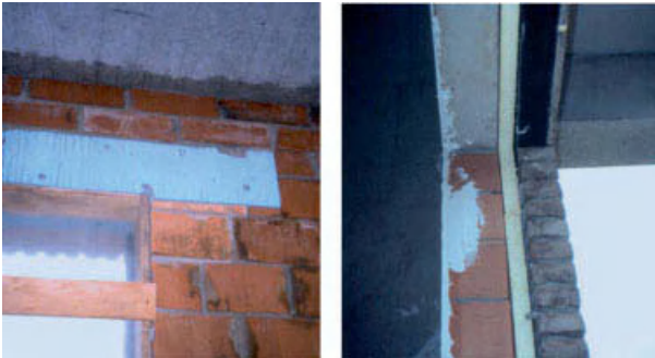
Figure 10.27. Lintels. On the left: how not to insulate, on the right: how to do it.
