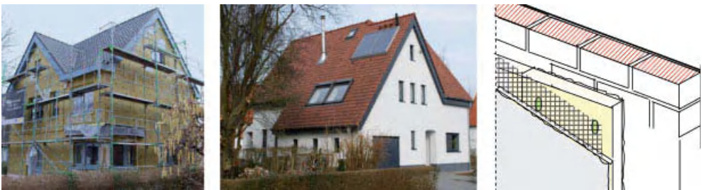
Figure 9.30. Massive walls with EIFS (on the left: while insulating, in the middle: once finished, on the right: a view of the assembly).
