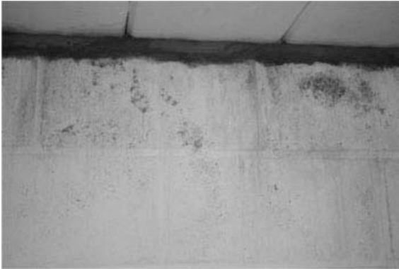
Figure 5.26. Outside protruding waterproof barrier below the floor at grade causes rain leakage into the basement.
