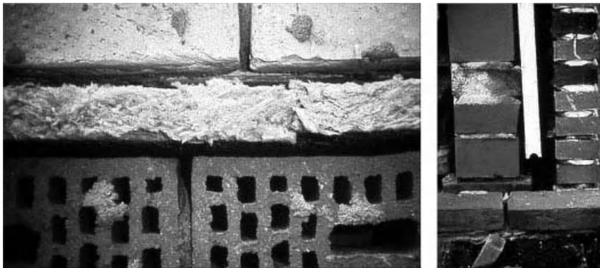
Figure 10.6. Insulation not linking up with the inside leaf (left), not touching the cavity tray (right).
