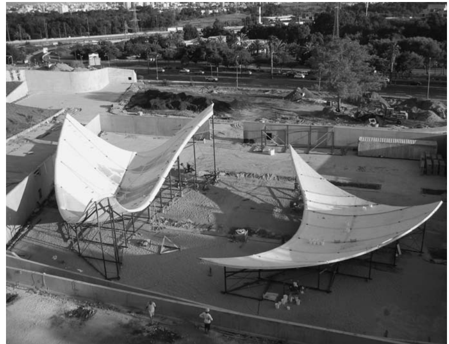
3.26 On site assembly and bonding of roof segments by Holland Composites Industrials.
