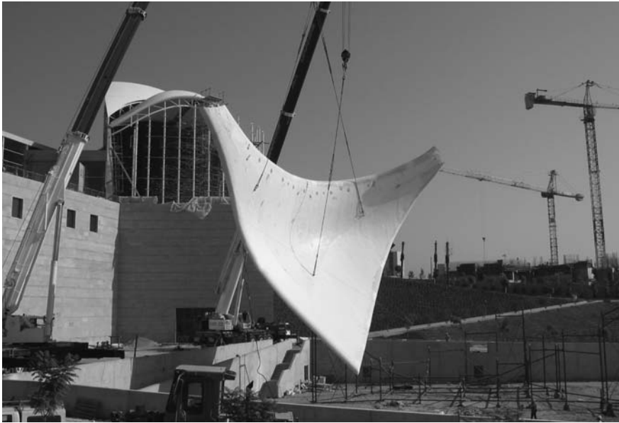
3.27 Installation of lower wing by Holland Composites Industrials and Octatube at Yitzhak Rabin Centre.
