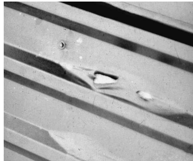
5.19 Delamination of outer paint finish due to safe temperatures being exceeded.
