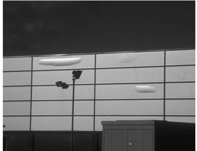
6.23 Typical example of delamination of composite panels.
