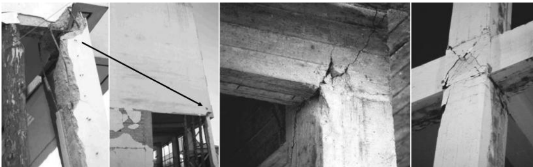
Figure 2.21 Shear failure of beam–column joints.
