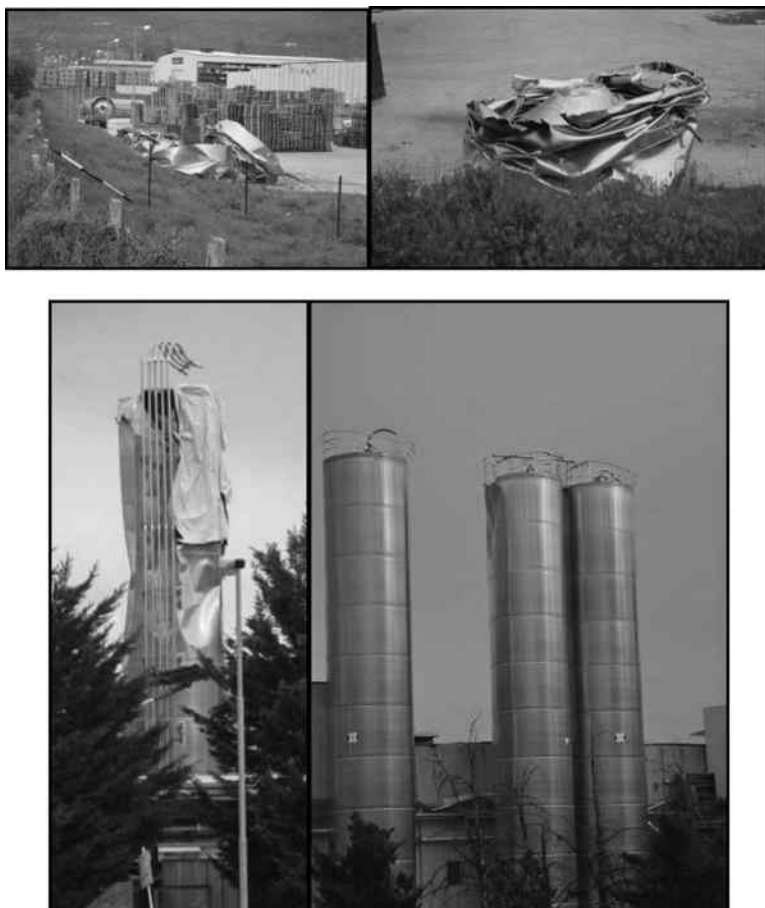
Figure 1.64 Local and global failure of silos.
