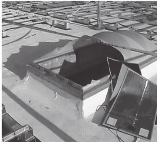
The skylight that the worker fell through
