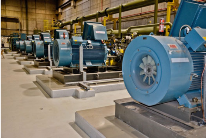
Fig. 11 Pumping station (Gorona del Viento, with permission)
