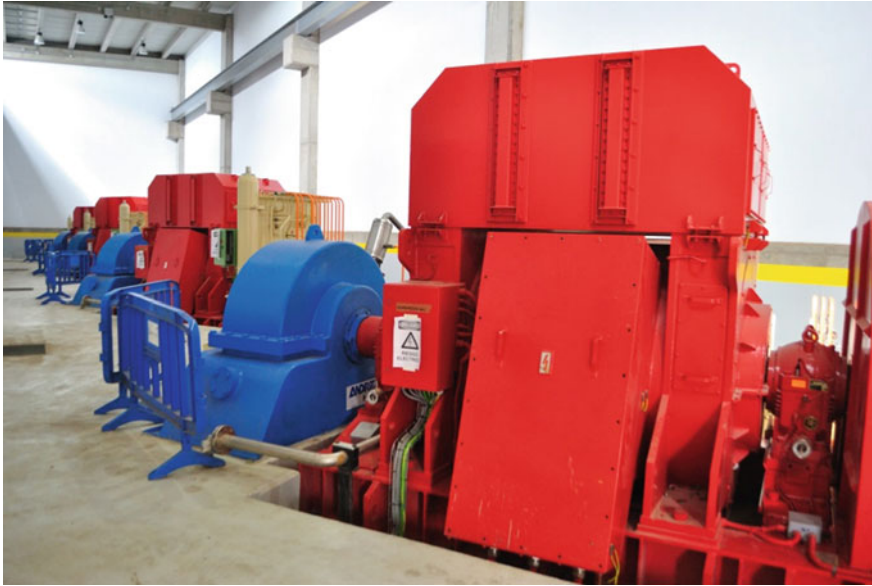
Fig. 13 Turbine station (Gorona del Viento, with permission)
