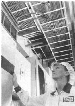
Figure 22.10 KHZ hot-dip galvanized cable ladder having oval rungs and closed rail profile meets Cadbury's stringent requirements at its Bournville factory (Wibe)
