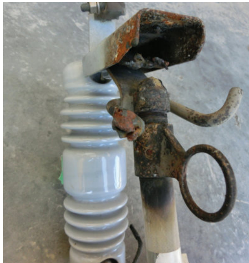
Figure 7.25 Cutout damaged by arcing in the field.
