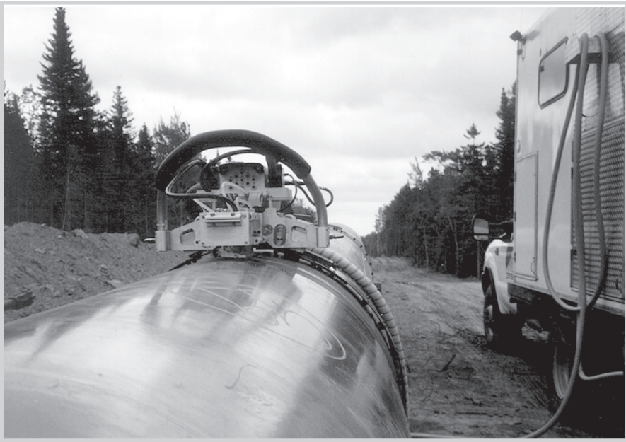
Fig. 13–8. Automated ultrasonic testing device clamped to the pipe. The same ultrasonic technology used in smart pigs is used to ensure weld quality during construction. (Courtesy Olympus NDT)
