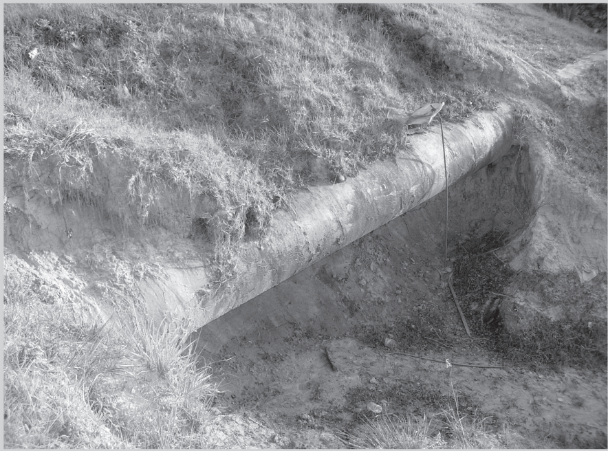
Fig. 9–6. Natural gas pipeline exposed by erosion (Courtesy Miesner, LLC)
