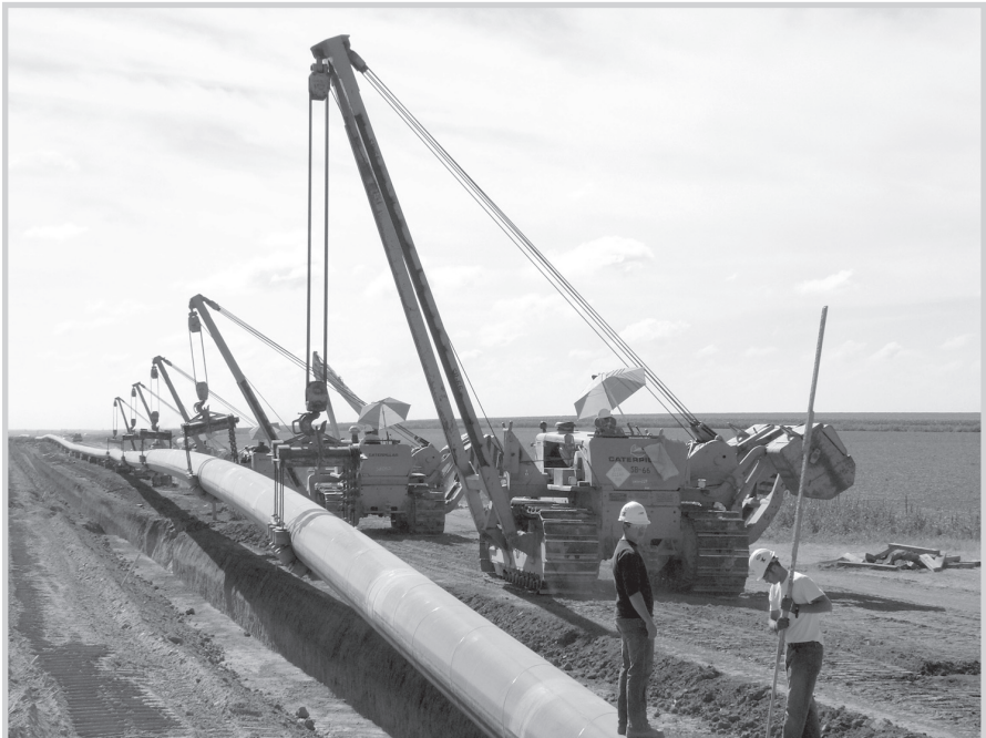
Fig. 13–11. Lowering in the pipeline (Courtesy U.S. Pipeline, Inc.; photo by Adam Aronson)
