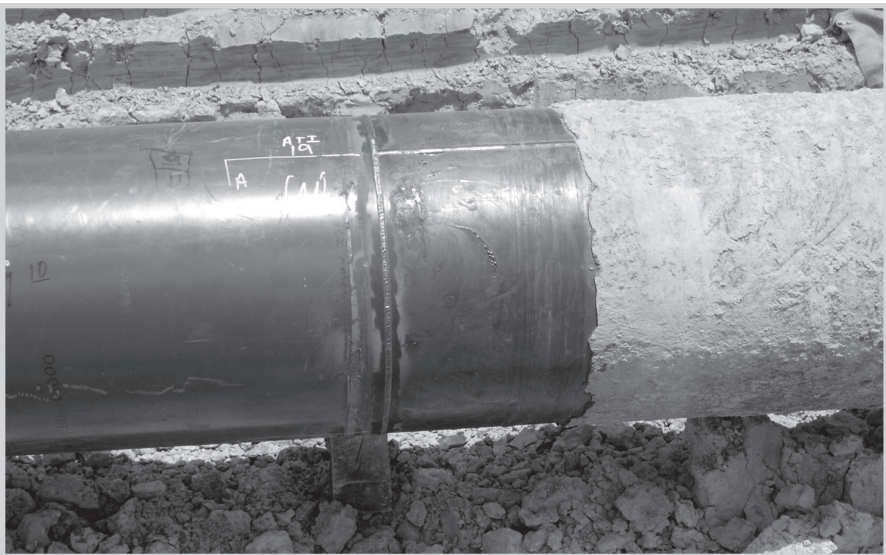
Fig. 11–2. Pipe with FBE coating welded to a pipe with coal tar enamel coating. The replacement pipe on the left is coated with FBE and welded to the older pipe on the right coated with coal tar. (Courtesy Miesner, LLC)
