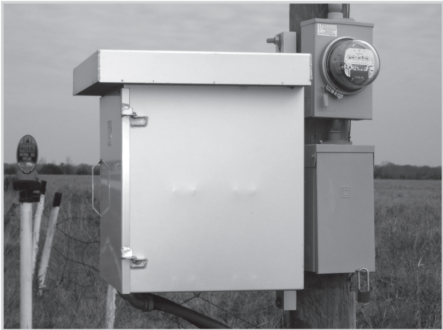
Fig. 9–13. Pipeline rectifier. Note the power meter and breaker box on the pole next to the rectifier and the line markers in the background. (Courtesy Miesner, LLC)
