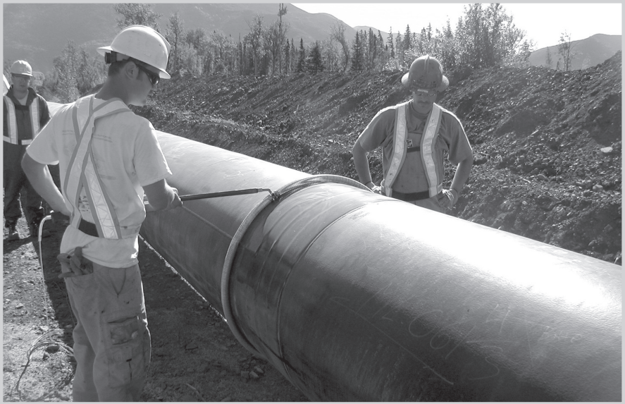
Fig. 13–10. Final inspection with a holiday detector. The detector produces an audible signal when it encounters a coating holiday. (Courtesy Canusa-CPS)
