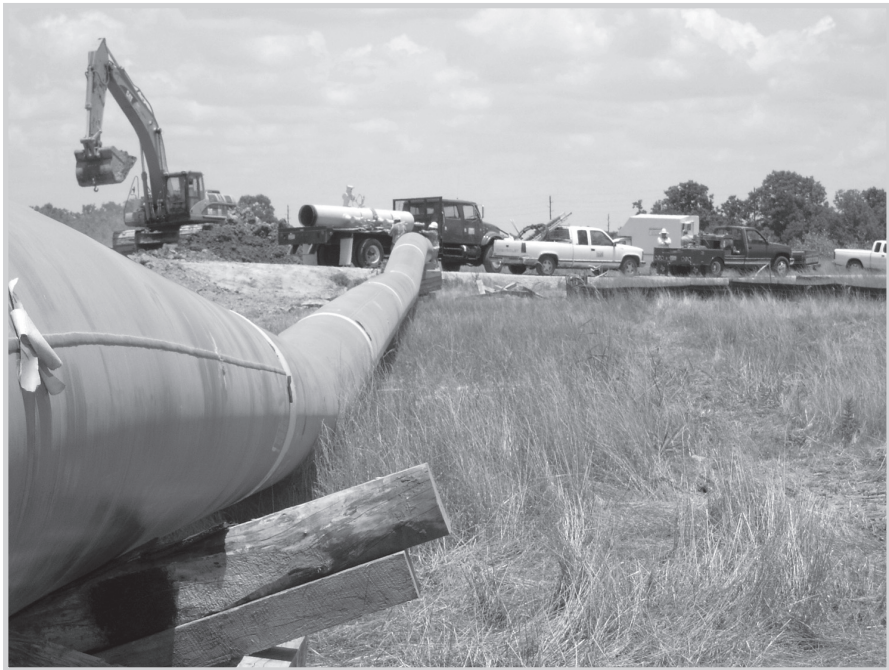
Fig. 13–13. Bent pipe stored for future use. A section of natural gas pipeline is bent to fit under a crude oil line. (Courtesy Miesner, LLC)
