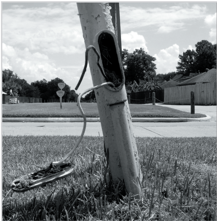
Fig. 9–29. Damaged cathodic test station (Courtesy Miesner, LLC)
