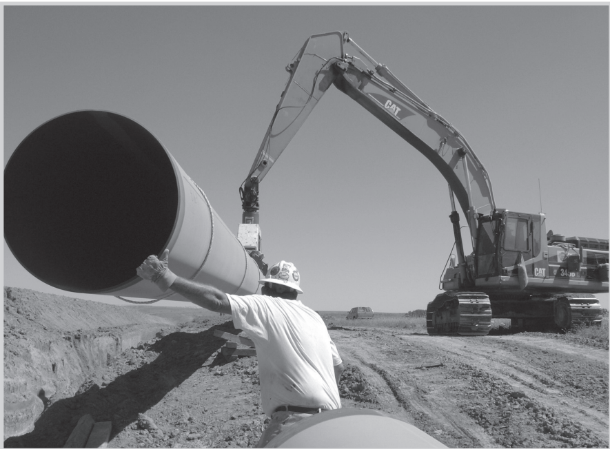
Fig. 13–2. Positioning pipe joints along the route. The pipe is hauled to the site by trucks, lifted off, and carefully placed into position prior to welding. (Courtesy U.S. Pipeline, Inc.; photo by Adam Aronson)
