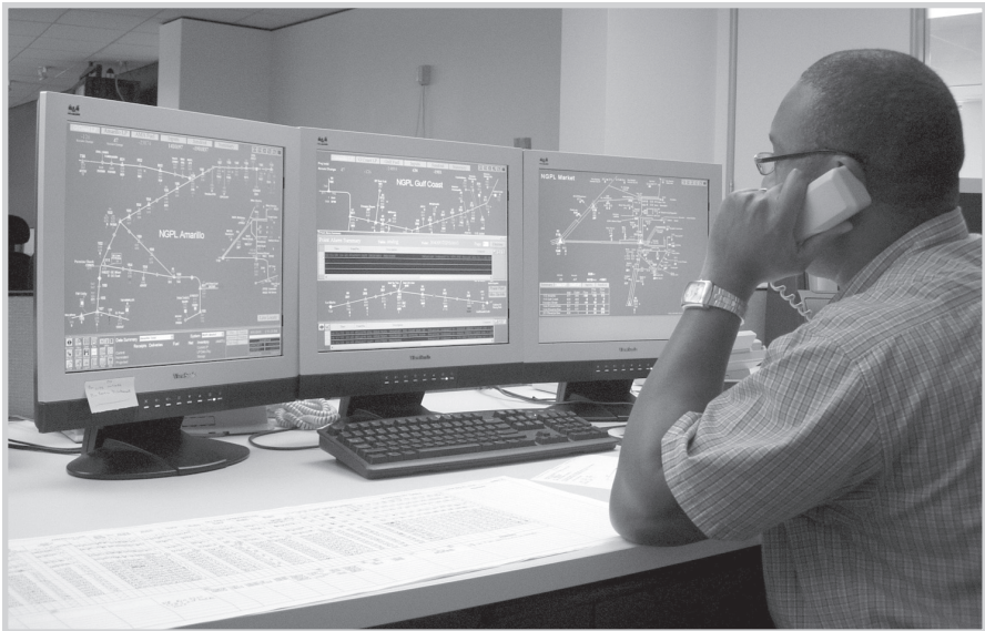
Fig. 5–14. Natural gas systems summary screens. The controller carefully considers the response to a message in the center of the middle screen. (Courtesy Kinder Morgan Gas Pipeline; photo by Tom Miesner)
