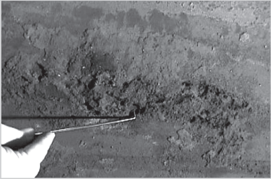
Fig. 9–3. Severe microbial corrosion (Source: National Transportation Safety Board)
