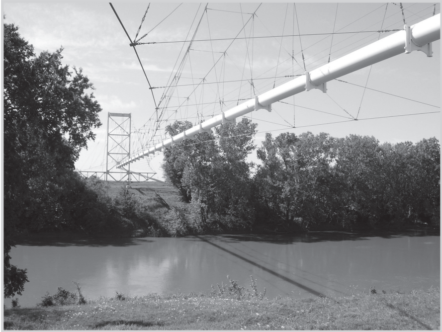
Fig. 13–14. Aerial crossing. A 30-in. natural gas pipeline crosses a small river. (Courtesy Miesner, LLC)
