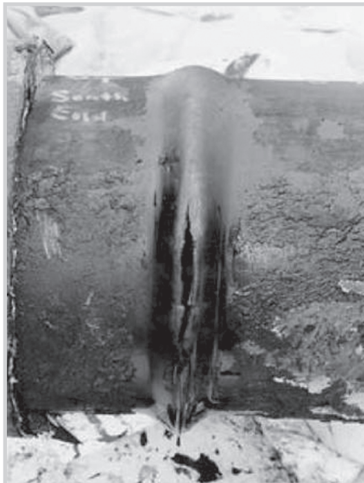
Fig. 9–9. Crack caused by buckling (Source: National Transportation Safety Board)
