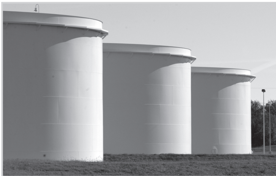
Fig. 12–18. Tank dikes. These dikes contain spills, keeping them from spreading and enabling quick cleanup. (Courtesy Explorer Pipeline Company)
