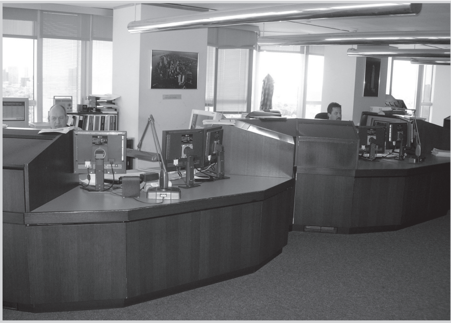
Fig. 5–12. Natural gas control room. (Courtesy Williams Gas Pipeline; photo by Tom Miesner)
