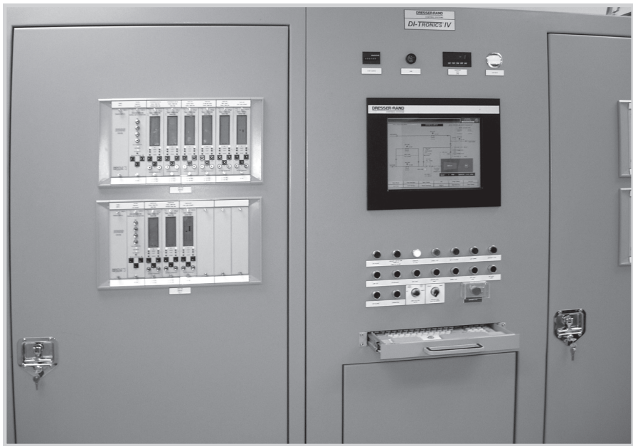
Fig. 8–6. Local station SCADA (Courtesy Williams Gas Pipeline; photo by Tom Miesner)
