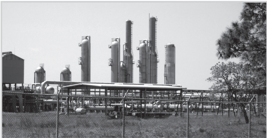
Fig. 5–3. Natural gas processing plant. The various towers each remove a specific type of hydrocarbon molecule from the stream. (Photo courtesy Miesner, LLC)
