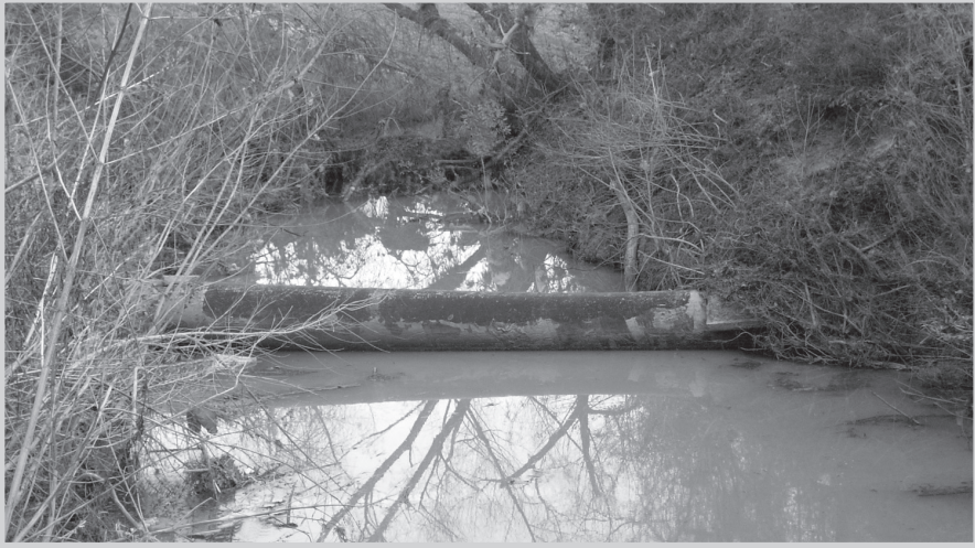
Fig. 9–7. Natural gas pipeline exposed in a drainage ditch (Courtesy Miesner, LLC)
