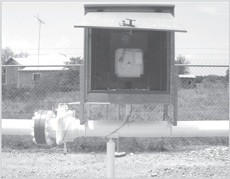
Fig. 5–6. Orifice meter run. An orifice plate is located in the pipe to the left of the box containing a paper chart. Note the white lines coming from the orifice plate to measure pressure. (Photo courtesy Miesner, LLC)
