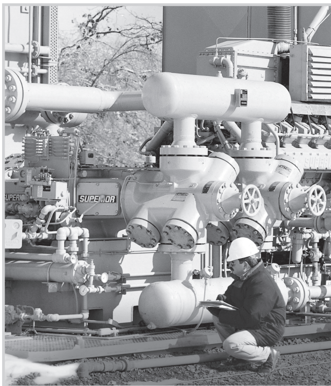
Fig. 11–22. Natural gas engine driving a reciprocating compressor. The engine is coupled to the compressor. (Courtesy Cooper Compression)
