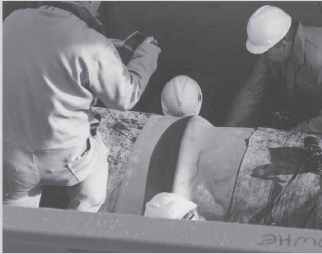
Fig. 9–8. Pipeline buckle caused by differential settlement through a landfill (Source: National Transportation Safety Board)
