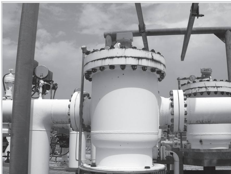
Fig. 11–6. Flanges welded to the pipe and bolted to a valve. Not visible between the flanges is a gasket of flexible material inserted to form a tight seal. (Courtesy Miesner, LLC)
