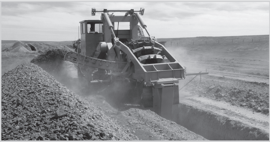
Fig. 13–9. Trenching machine. Soil from the trench is placed on one side of the ditch. The other side is used for construction activities. (Courtesy U.S. Pipeline, Inc.; photo by Adam Aronson)
