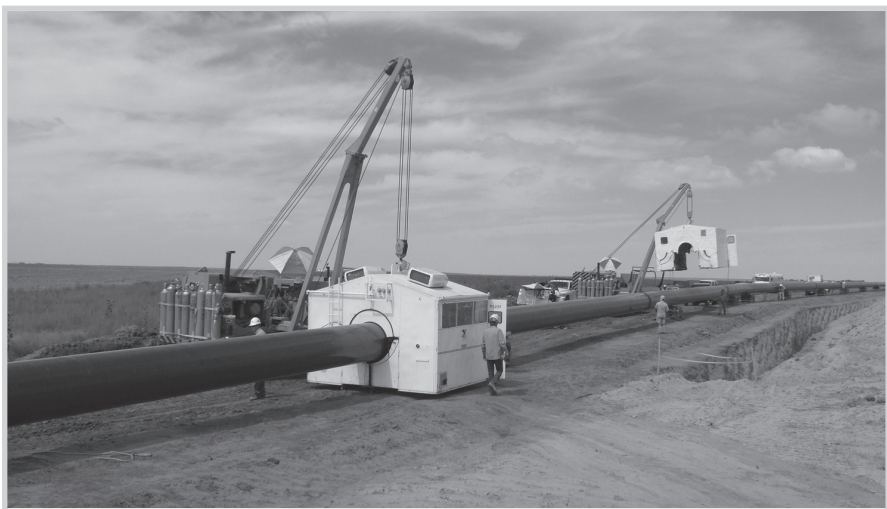
Fig. 13–3. Welding tents. Tents are sometimes used to cover the pipe and improve welding or working conditions. (Courtesy U.S. Pipeline, Inc.; photo by Adam Aronson)
