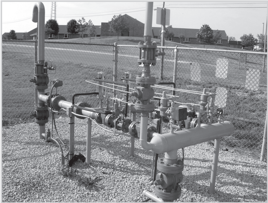
Fig. 5-11. City gate station to a town along the route (Photo courtesy Miesner, LLC)
