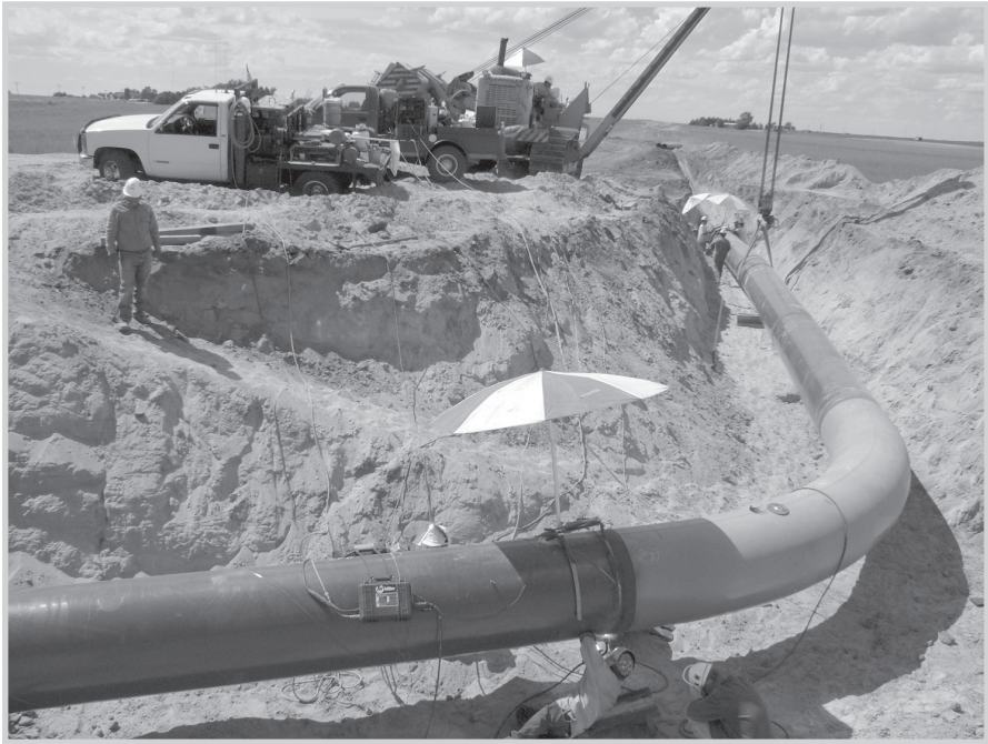
Fig. 13–16. Welder tying in a bend (Courtesy U.S. Pipeline, Inc.; photo by Adam Aronson)
