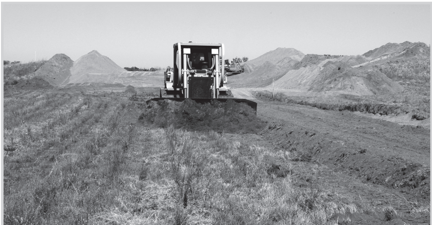
Fig. 13–1. Stockpiling topsoil. Topsoil is stripped from the right-of-way, stored in piles, and put back when the pipeline is complete. (Courtesy U.S. Pipeline, Inc.; photo by Adam Aronson)
