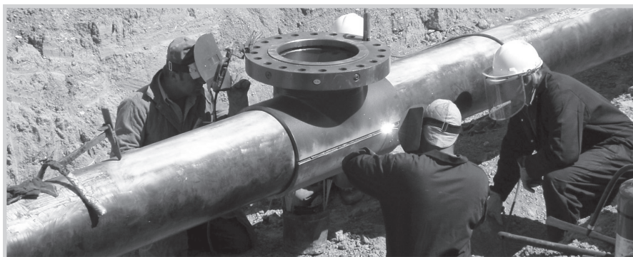
Fig. 9–24. Welding a hot tap fitting onto the line (Photo by Frank Gonzales)
