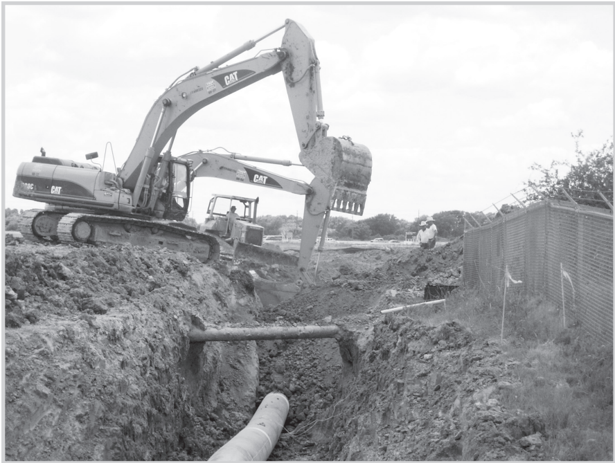
Fig. 13–12. Backfilling the trench. The bulldozer and front backhoe fill the trench, and the one in back compacts the backfill. Another pipeline sits in the middle of it all. (Courtesy Miesner, LLC)
