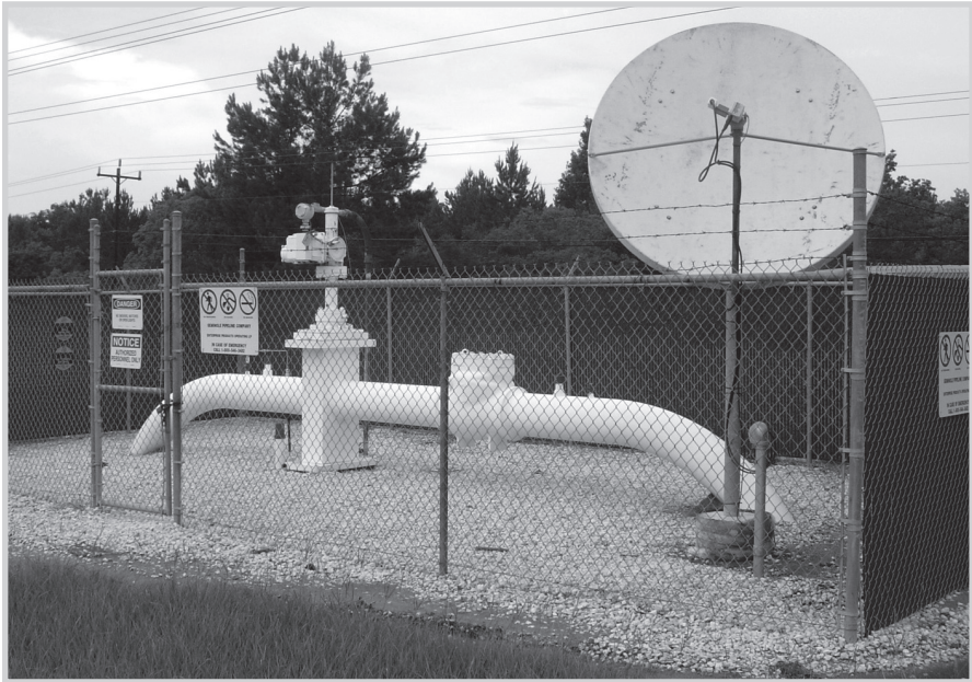
Fig. 8–3. Block valve with satellite communications (Courtesy Miesner, LLC)
