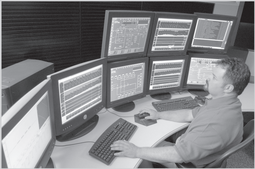
Fig. 4–3. Oil pipeline controller at work. Each display shows different aspects of pipeline operation. (Courtesy Explorer Pipeline Company)
