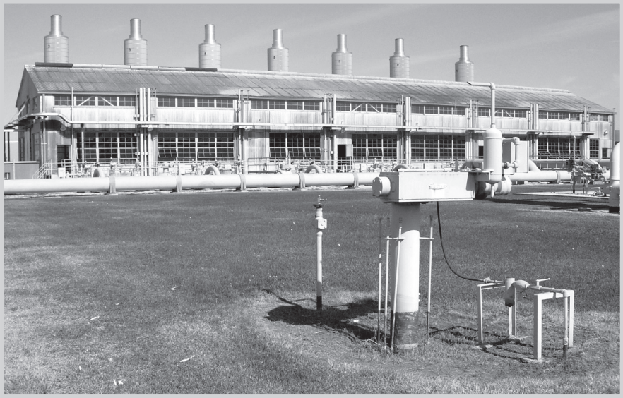
Fig. 5–8. Origination gas compressor station. Several gathering lines from onshore and one from offshore enter this mainline origination compression station. The natural gas is aggregated into a common suction header, and a combination of the seven reciprocating compressors, driven by natural gas–fired reciprocating engines, add pressure to the gas before it is discharged into a 30-in. natural gas main line. (Courtesy Williams Gas Pipeline; photo by Tom Miesner)
