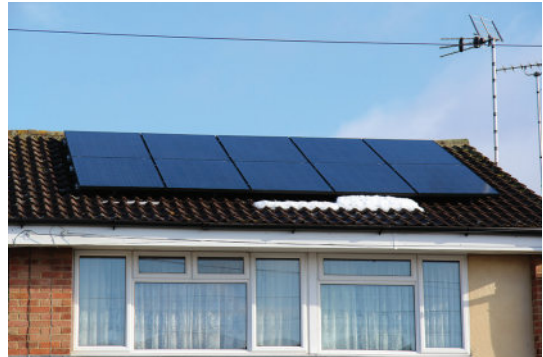
Figure 7.26 A 4kW array of PV panels (ten front and six more at the back)
