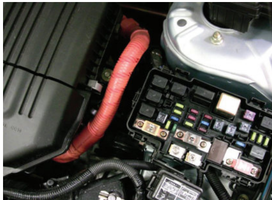
Figure 9.49 Power cable connected to the motor (remember, orange cables are high voltage)
