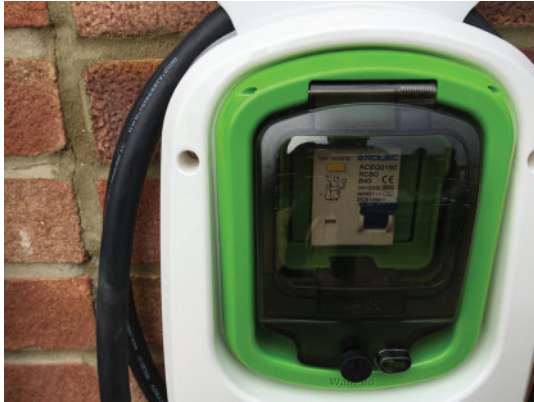
Figure 7.29 Domestic wall box mounted outside, with a permanent cable attached. It includes a residual current circuit breaker
