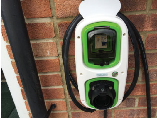
Figure 7.4 Domestic charging point
