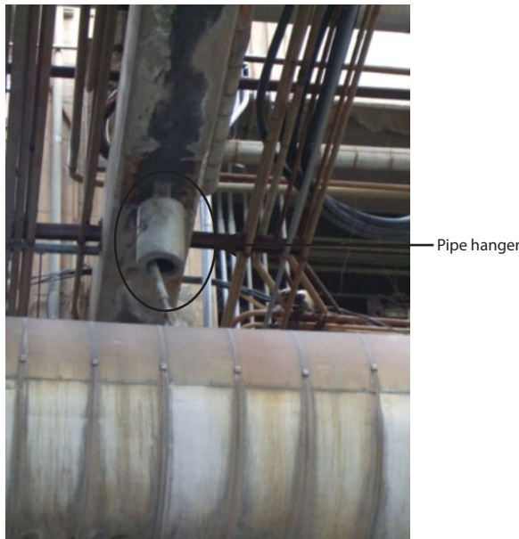
Figure 13.5 Broken pipe hanger support.
