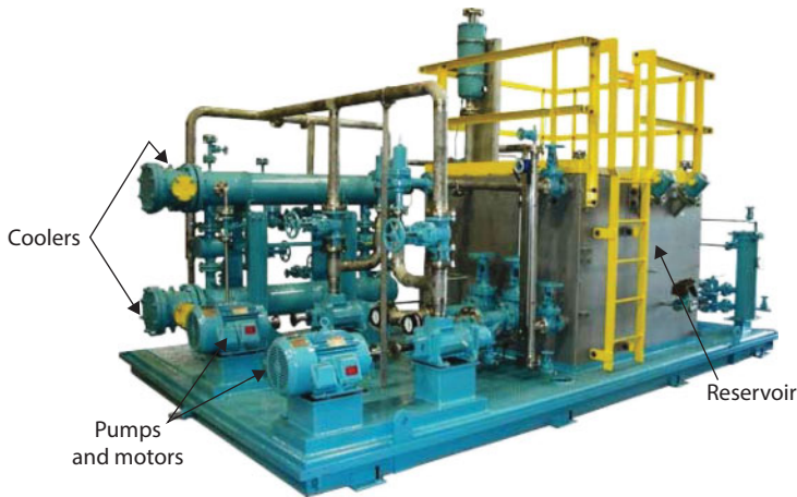
Figure 2.19 Complex forced lubrication system with pumps, reservoir in blue, coolers, extraction fans on top of reservoir.
