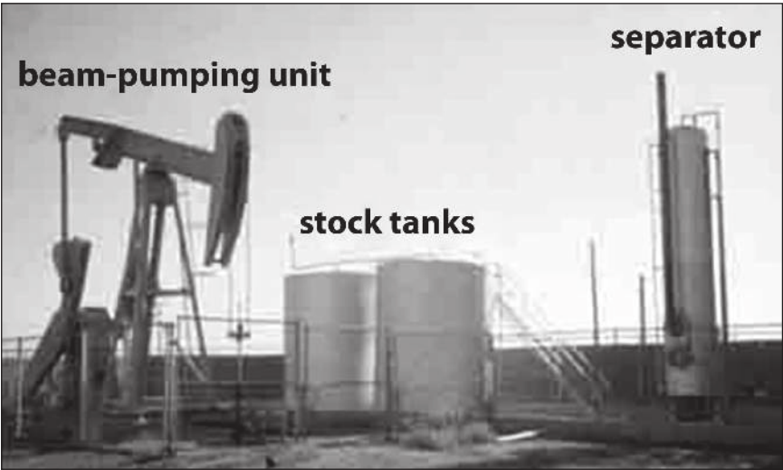
Plate I-1. Oil well with separator and stock tanks
