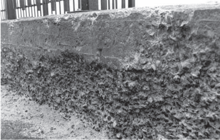
Figure 11.7 Scaling on a wall exposed to de-icing salts during winter. In addition to architectural damage, severe scaling can lead to progressive structural deterioration.
