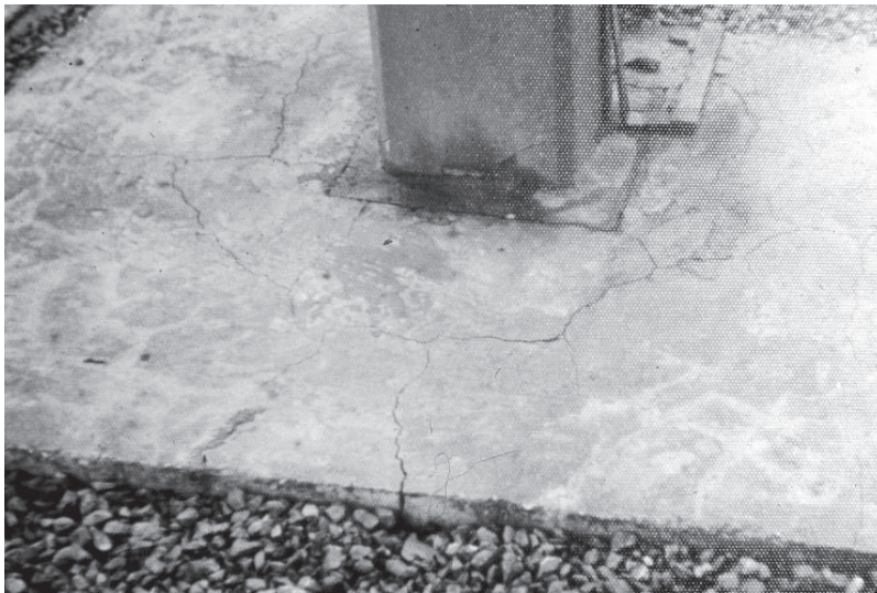
Figure 13.11 Concrete bases in Plymouth, Devon: first identified case of ASR in the UK.
