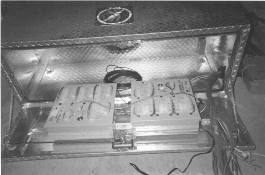
14.13 Datalogger installed on Portage Creek Bridge.
