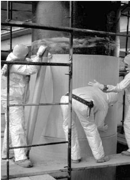
2.4 Use of wet layup for installation of a fiber-reinforced polymer jacket for seismic retrofit of columns.
