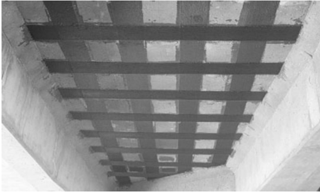
2.5 External bonding of fabric onto deck soffits for strengthening using wet layup.
