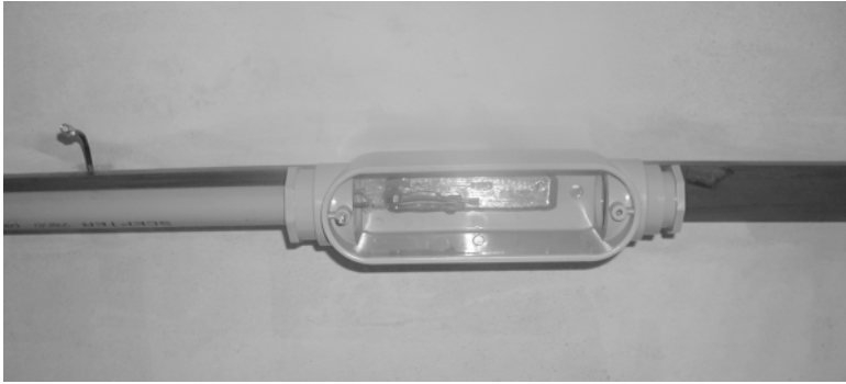
14.7 Rigid polyvinyl chloride conduit and junction box for externally installed gauges.
