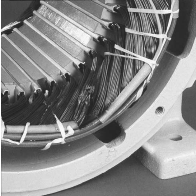
FIGURE 8.19 Winding damaged by voltage surge.
