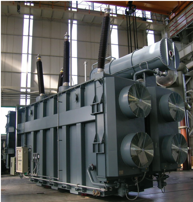
Fig. 2.22. Large three-phase oil cooled power transformer with external air blowers.
