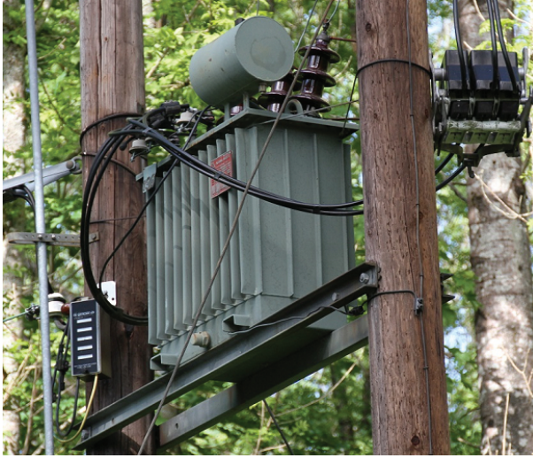
Fig. 2.21. Three-phase distribution transformer.
