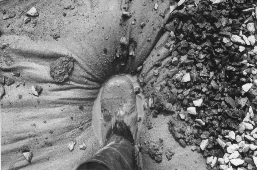
7.1 Non-woven geotextile over soft soil as a separator for crushed stones and a worker's boot.
