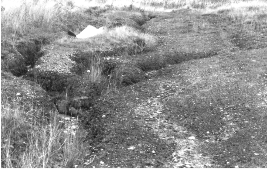
12.9 Eroded surface of a waste tip (note the sparseness of the vegetation).
