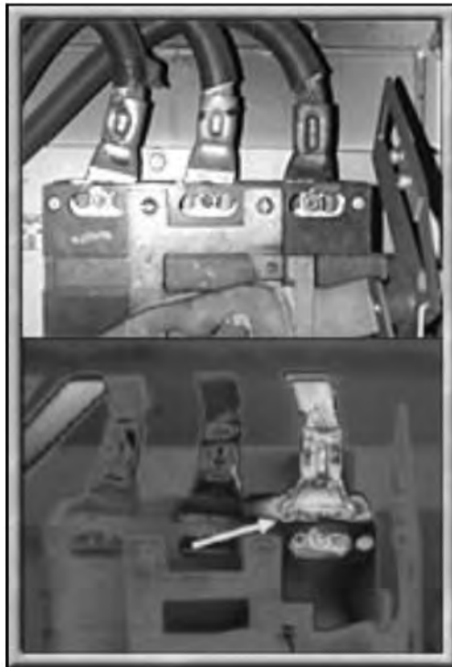
Figure 8.3 Resistive heating at an electrical connection (source: www.cinde.ca)
