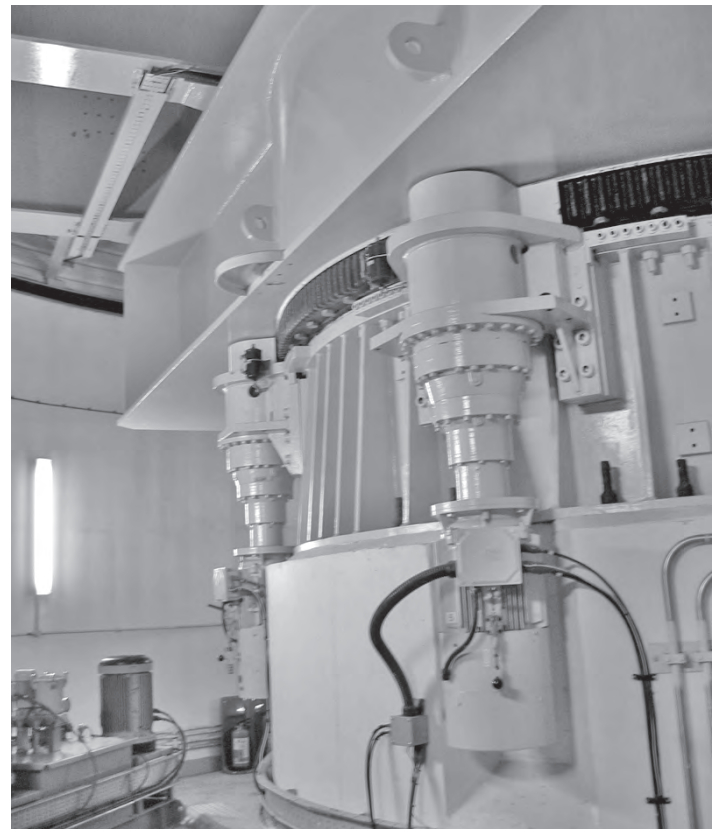
Figure 16.38 Drive motors at Selby Swing Bridge (photograph courtesy of R Evans)
