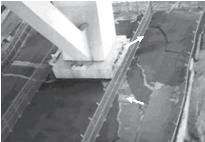
Figure 6.4 Soil boils and cracks at pier foundations of Nishinomiya-ko Bridge in the 1995 Kobe (Japan) earthquake (courtesy of USGS)
