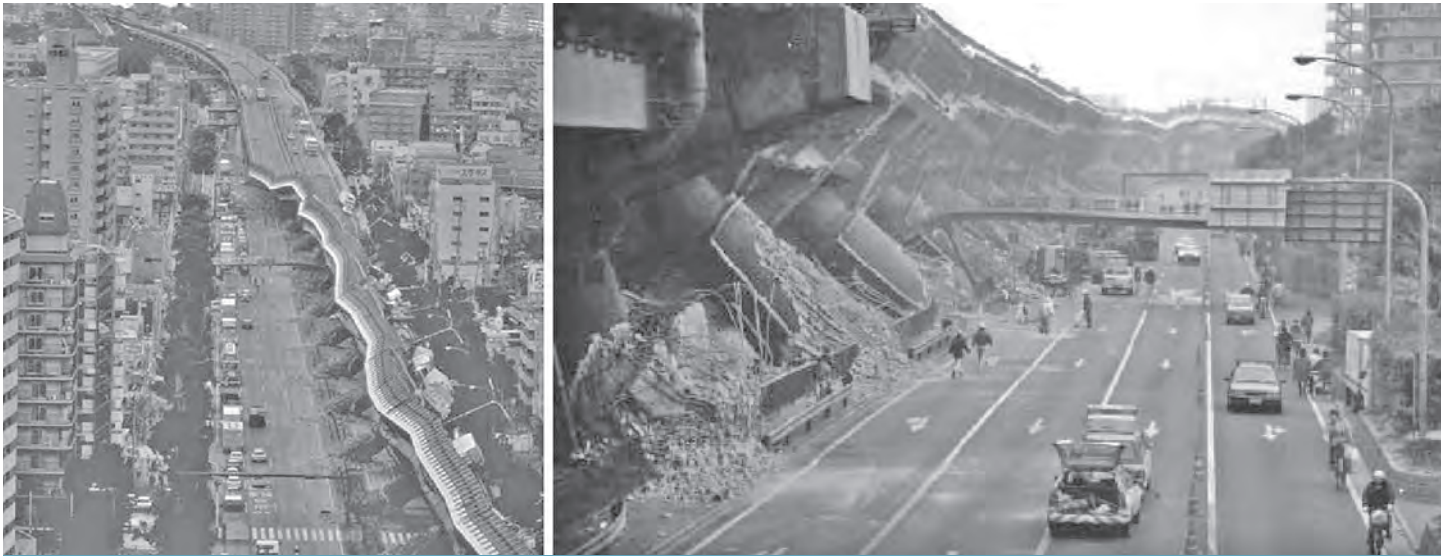
Figure 6.2 Collapse of the Hanshin Expressway elevated road, Hyogo-ken Nanbu (Japan) earthquake of 17 January 1995 (courtesy of National Information Service for Earthquake Engineering, University of California, Berkeley)
