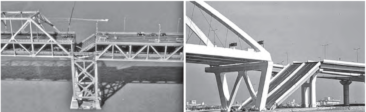
Figure 6.7 Damage by unseating at joints: left, the Oakland Bay Bridge failed span in the Loma Prieta (USA) earthquake; right, the Nishinomiya bridge collapse during the Hyogo-ken Nanbu (Japan) earthquake (courtesy of USGS)
