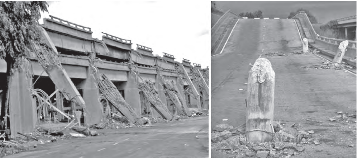
Figure 6.6 Damage to substructure resulting from the Loma Prieta (USA) earthquake of 17 October 1989: left, the Cypress Street Viaduct (I-880); right, failure of the piers of the Struve Slough Bridge (courtesy of USGS)
