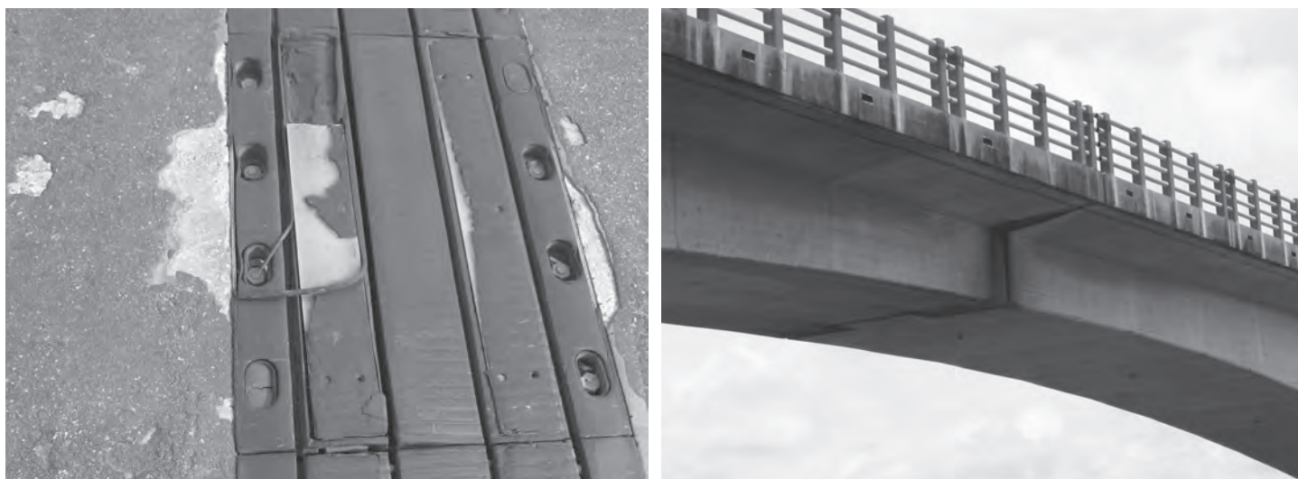
Figure 22.5 (a) Failure of expansion joint in road bridge; (b) associated leakage of water through the unprotected half-joint (these photographs were taken less than 6 years after the bridge was first opened to traffic)
