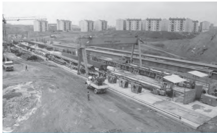
Figure 9.10 Casting bed for pre-tensioned beams
