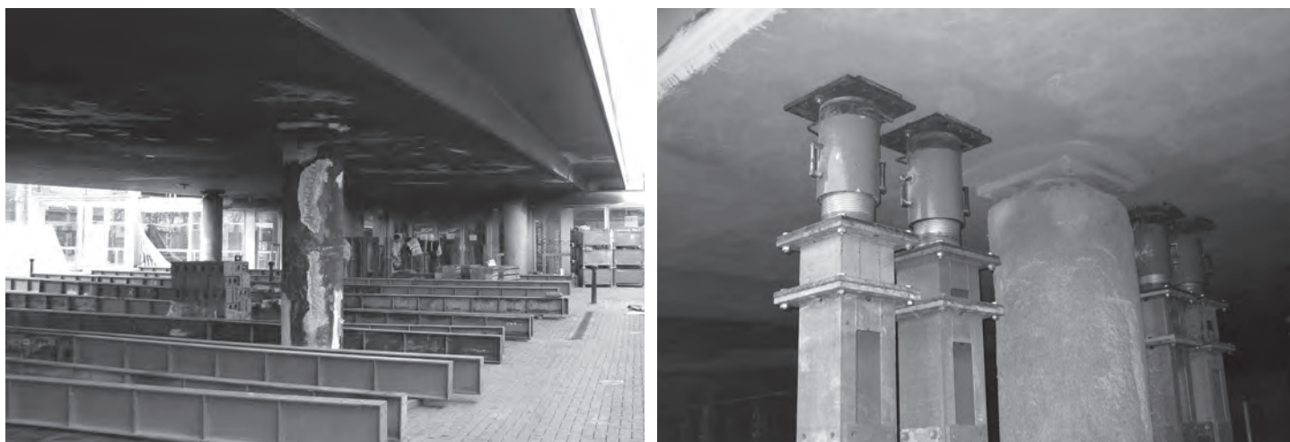
Figure 26.1 (a) Fire damage to concrete viaduct (left) and (b) concrete repairs with temporary jacking for bearing replacement (photographs courtesy of Jacobs)
