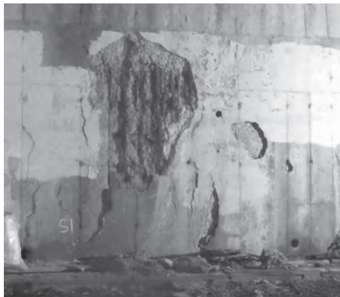
Figure 25.1 Concrete spalling (courtesy of Yellowstone National Park)
