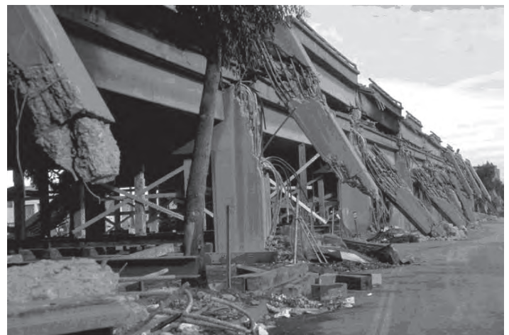
Figure 5.21 Freeway bridge collapse due to earthquake, October 17, 1989, Loma Prieta, California, (courtesy of US Geological Survey)
