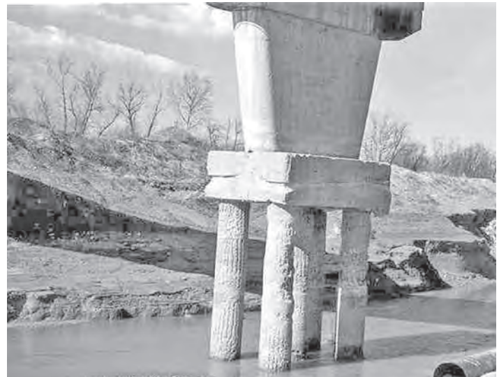
Figure 3.40 Example of scour (courtesy of Department of Transport)
