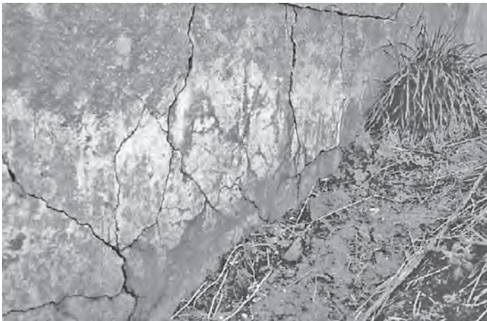
Figure 24.4 Destructive sulphate reaction, causing cracking in concrete (photograph courtesy of LCPC)
