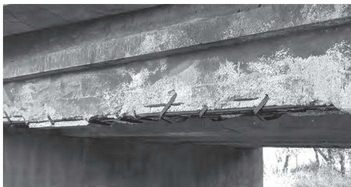
Figure 25.6 Concrete deck defects
