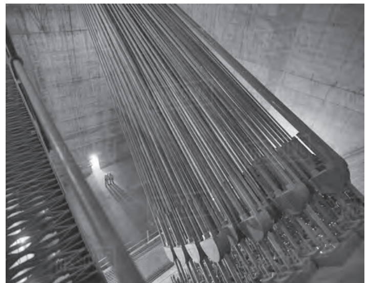
Figure 15.33 Strand divergence in anchor chamber
