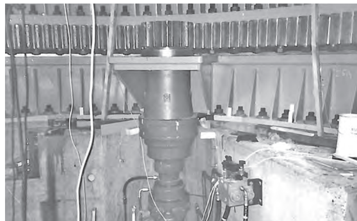
Figure 16.35 Drive motor inside pivot pier of Næstved Swing Bridge (image courtesy of the Danish Road Directorate)
