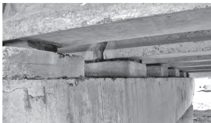
Figure 20.18 Lack of provision for jacking: detail (reproduced with permission © the Highways Agency)
