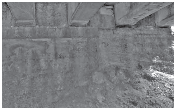
Figure 20.16 Lack of provision for jacking (reproduced with permission © the Highways Agency)
