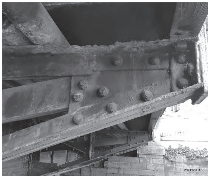
Figure 25.9 Corrosion of a steel truss and plates on the Oakland Bridge (courtesy of Oregon Department of Transportation)
