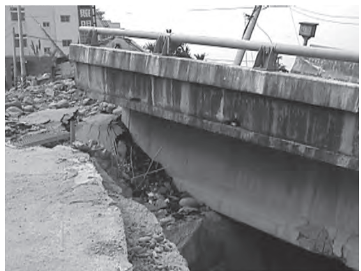
Figure 6.9 Failure of the abutment of the Highway 3 North-East out of Fengyuan during the 1999 Chi-Chi earthquake in Taiwan (courtesy of National Information Service for Earthquake Engineering, University of California, Berkeley)
