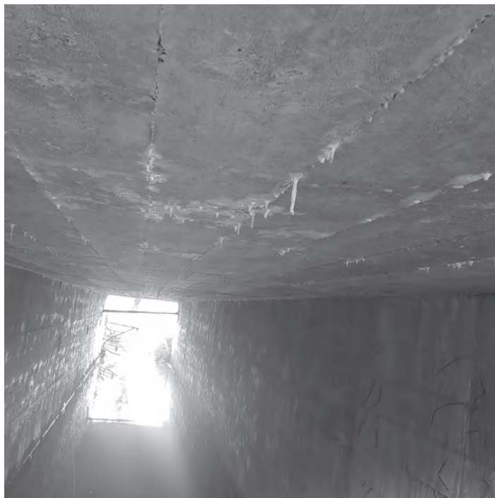
Figure 25.8 Water leakage through deck soffit cracks
