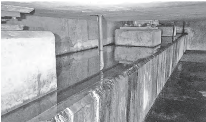
Figure 22.4 Raised plinth for protection of bridge bearing: the water ponding around the raised plinth is the result of inadequate design or maintenance of the drainage outlet, which has become blocked with debris (this photograph was taken less than 6 years after the bridge was first constructed)
