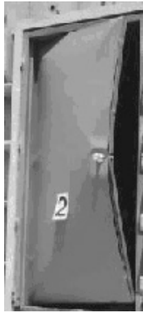
FIGURE 10.21: Conventional Hollow Metal Door Damage Under Low Blast Load
