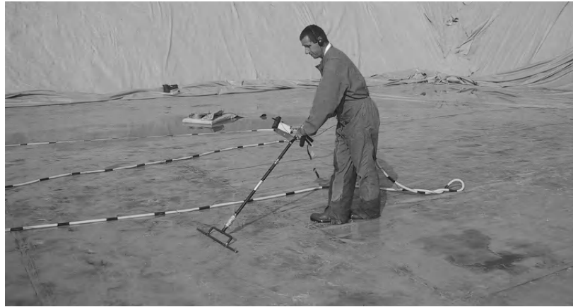
Figure 10.22. Leak detection device in the formation level of a waste storage site [CAQ 06].
