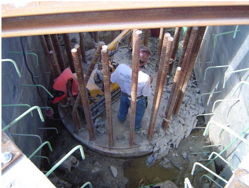
Figure 5.4.3.3-1 Precast Concrete Pier Box Cofferdam Top photo: Exterior View Bottom Photo: Interior View (source: Cardi Corporation)
