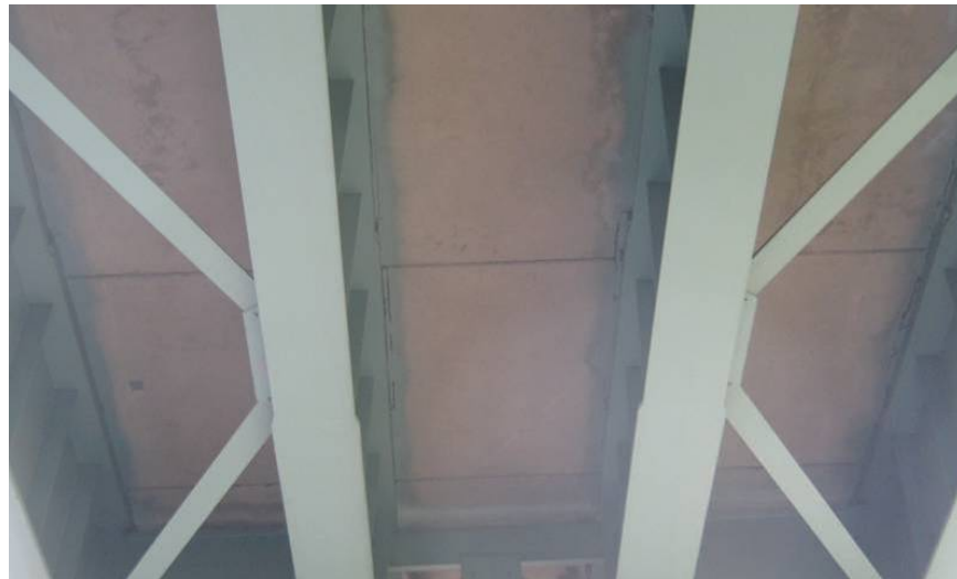
Figure 8.2.1.2-2 Underside of Bridge 03200 after 19 Years in Service
