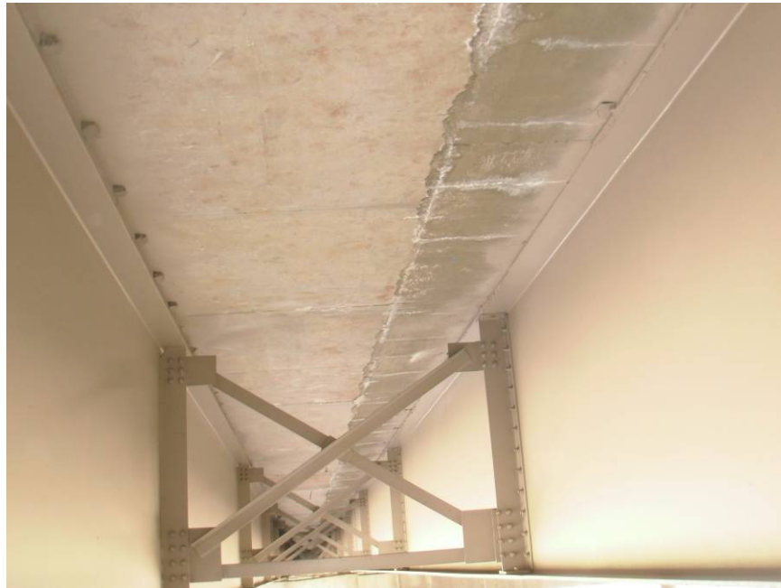
Figure 7.8-1 Cracking in Closure Pour Concrete
