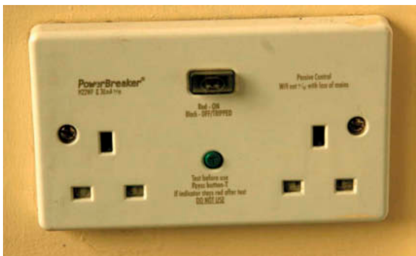
Figure 5.34 RCD socket outlet
