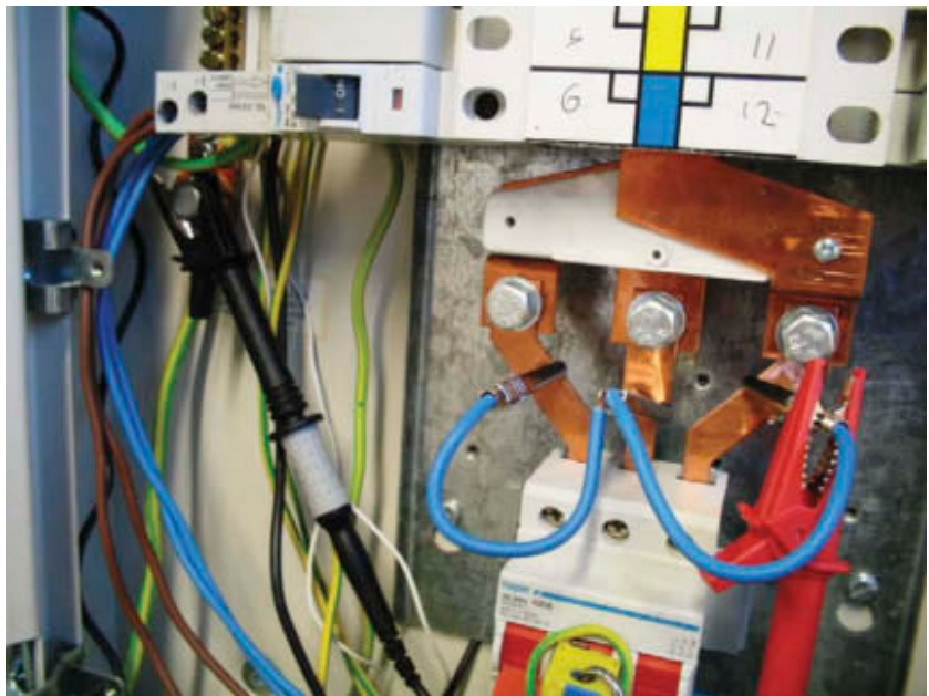
Figure 4.53 Test line to earth
