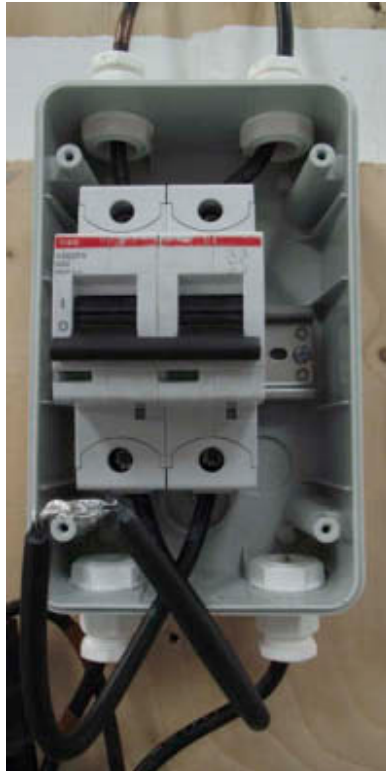
Figure 10.13 D.C. cables linked
