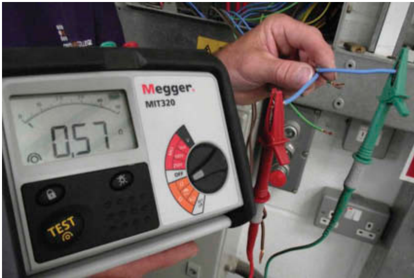
Figure 4.34 Test each end of the neutral conductor
