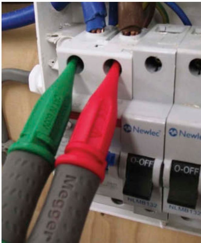
Figure 5.25 Test between incoming line and neutral
