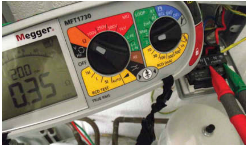
Figure 4.26 Probes on line and earth
