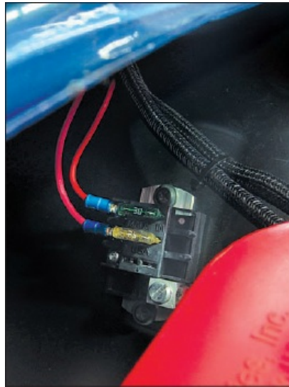
Fig. 5.60. I connected the heavy red 12 AWG power wire from the Digital 6AL to the fuse panel and fused it with a 25-amp fuse.
