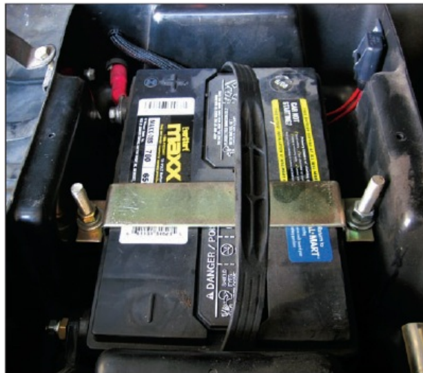
Fig. 6.46. Bill must have bumped his head just before choosing a battery with side-post terminals only. No matter; I keep adapters on hand to make correct connections to the side posts. I also mounted the fuse holder in the battery box.
