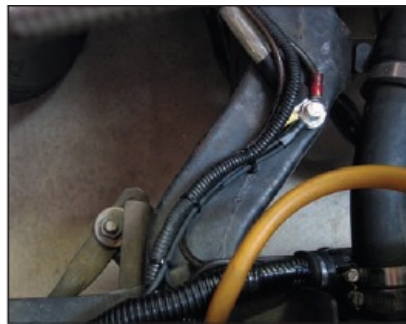
Fig. 4.10. I grounded the fans at the main ground location on the frame rail, which includes the ground upgrade for the alternator. The return path from the fans to the alternator is very short.
