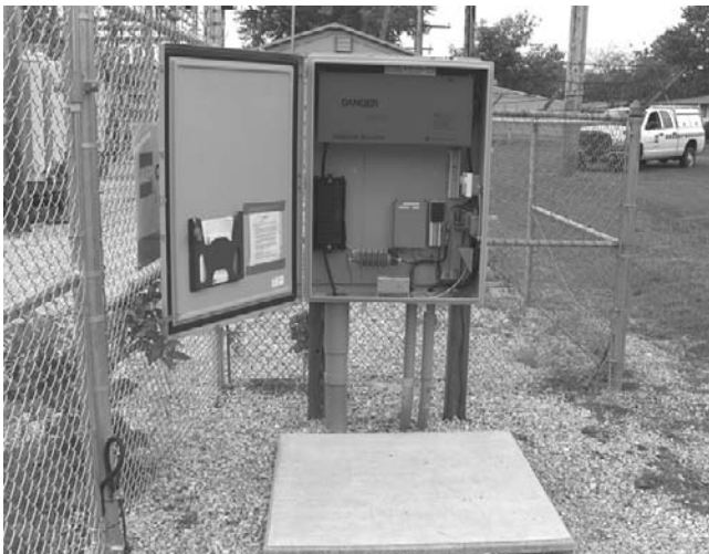
Figure 6.19 Station copper HVI.
