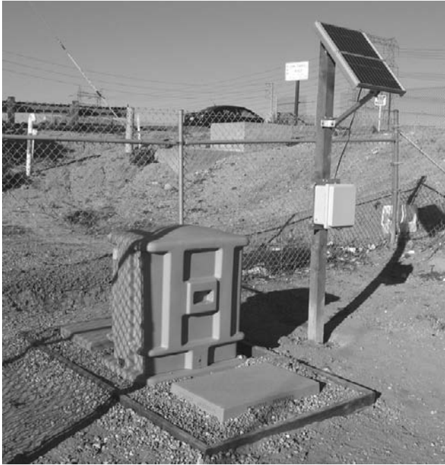
Figure 6.24 CFJ fiber—with solar power. Courtesy of RLH Industries, Inc.
