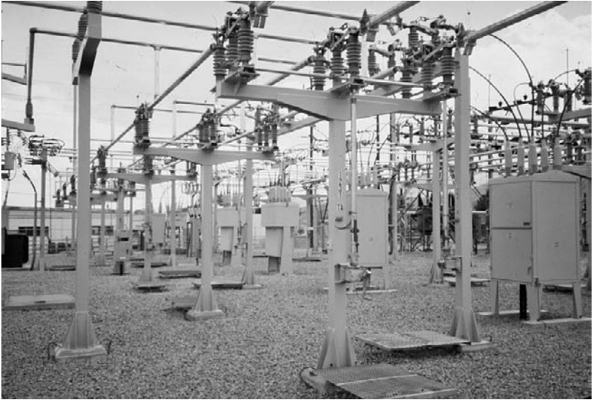
Figure 2.13 Typical distribution substation.
