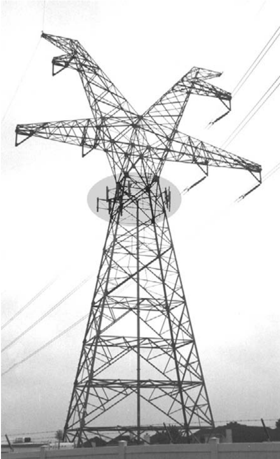
Figure 6.29 Wireless cell site on power transmission tower.
