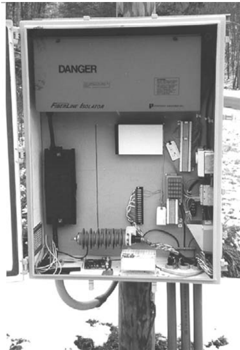
Figure 6.20 Station copper HVI—pole mount.
