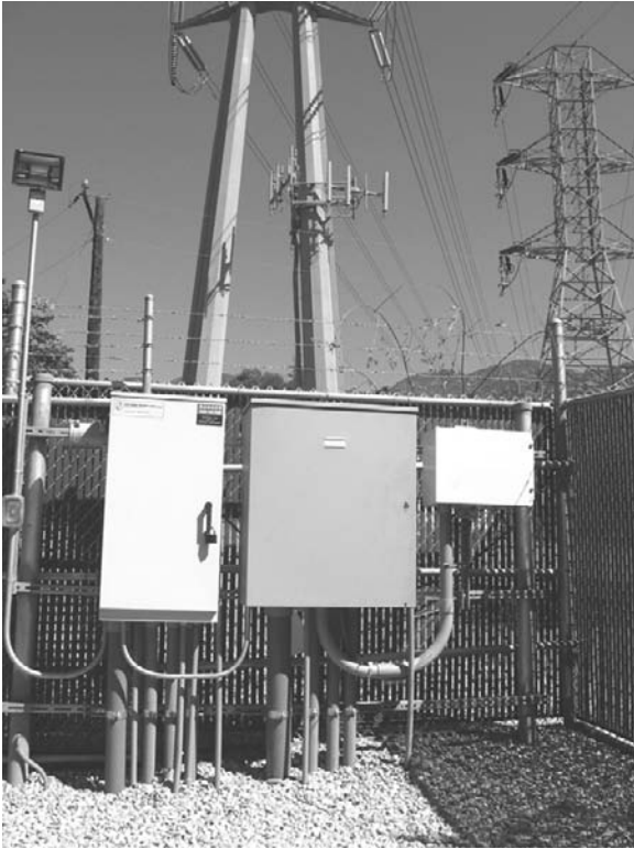
Figure 6.27 OEI—wireless cell site on power tower. Courtesy of RLH Industries, Inc.
