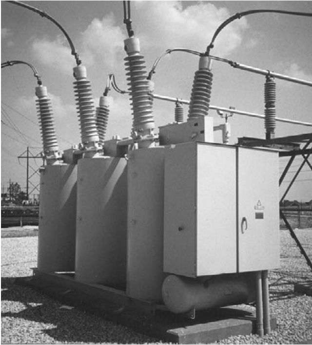
Figure 2.17 A 138 kV oil circuit breaker.
