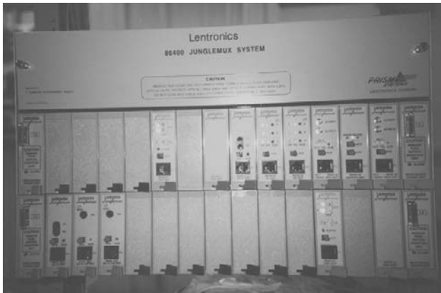
Figure 4.1 Transfer trip equipment.
