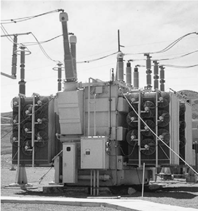
Figure 2.15 Power transformer 345 kV/120 kV.
