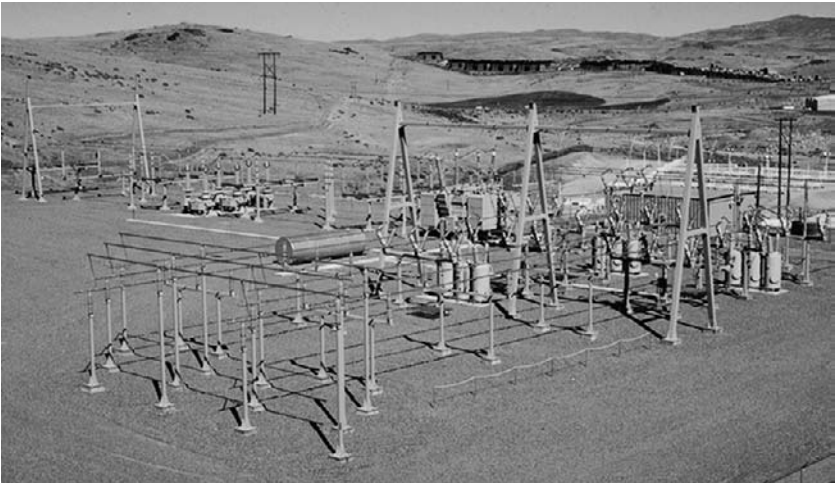
Figure 2.14 Typical transmission substation.
