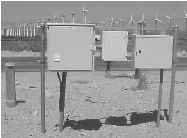
Figure 6.26 CFJ fiber wind farm-2. Courtesy of RLH Industries, Inc.
