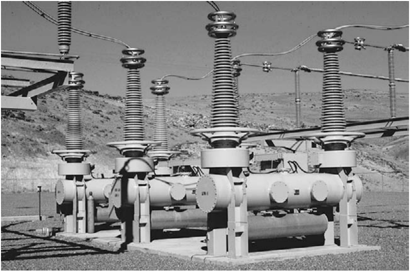
Figure 2.16 Gas circuit breaker 345 kV.
