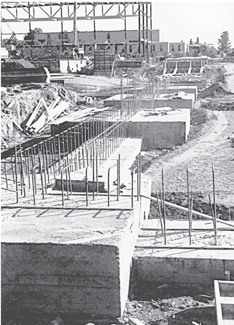
FIGURE 10-2 Column and wall footings. The Health, Physical Education and Recreation Complex, Hudson Valley Community College, Troy, New York. (George Limbrunner)
