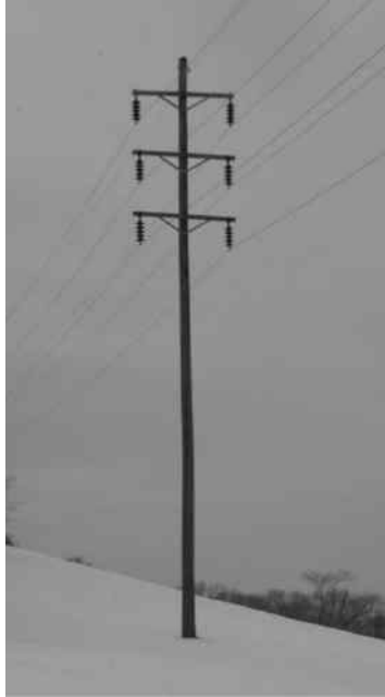
FIGURE 2.6 Medium-voltage distribution tower. (Photograph by author.)
