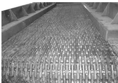
FIGURE 7.16 Typical chain grate.
