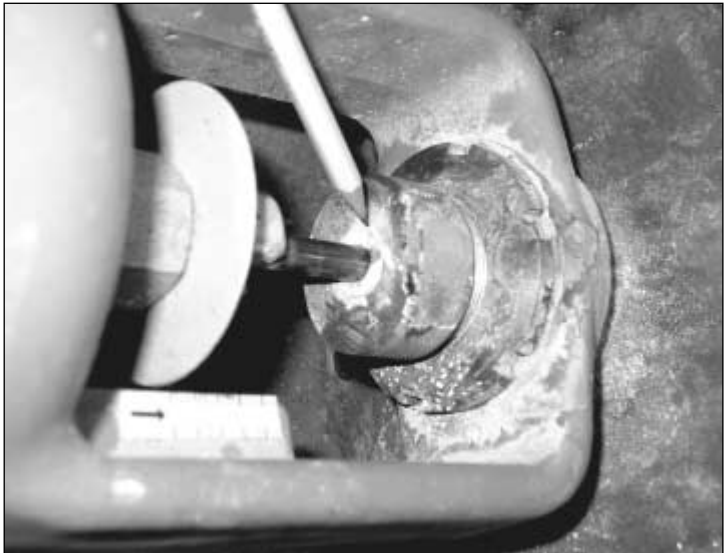
FIGURE 12.18 Corrosion on steam valve from leaking valve seal.
