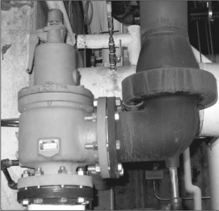
FIGURE 12.3 Steam pop-off valve (rated at 30 psi).
