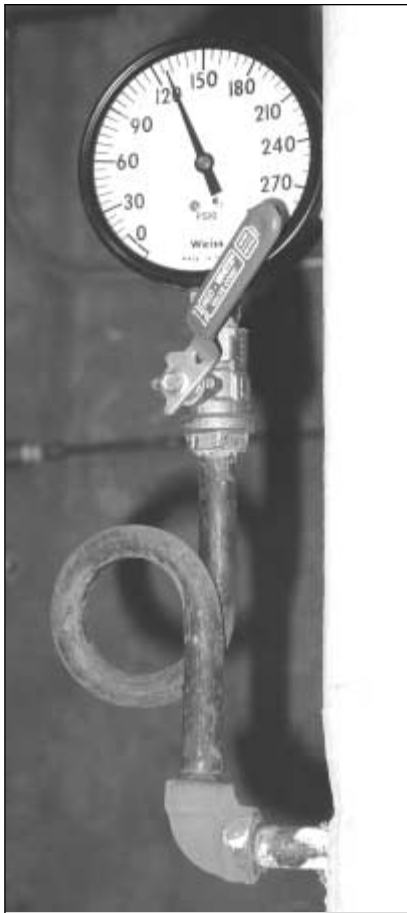
FIGURE 12.16 Steam pressure gauge with protective loop.
