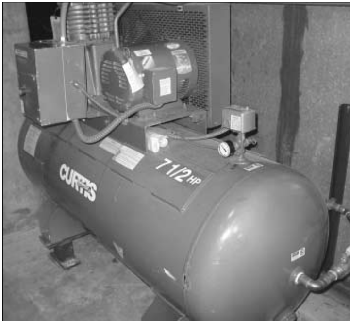
FIGURE 2.14 Combined air compressor and storage tank.
