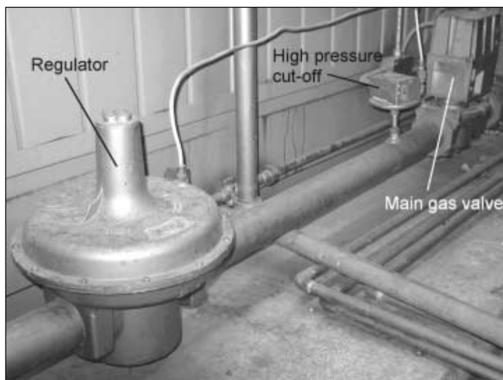
FIGURE 11.8 Boiler gas valve and high pressure cut-out.
