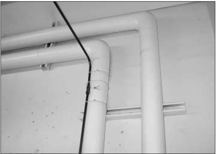
FIGURE 3.2 Insulated pipe mounted on wall brackets.
