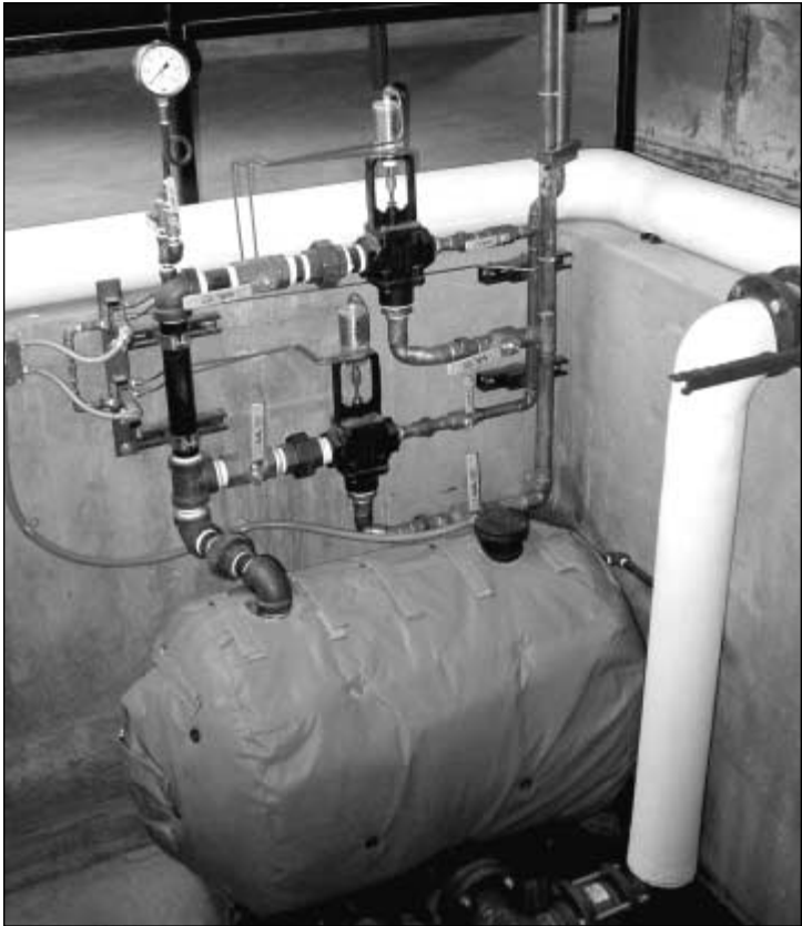
FIGURE 12.12 Condensate receiver tank, air-pump driven.
