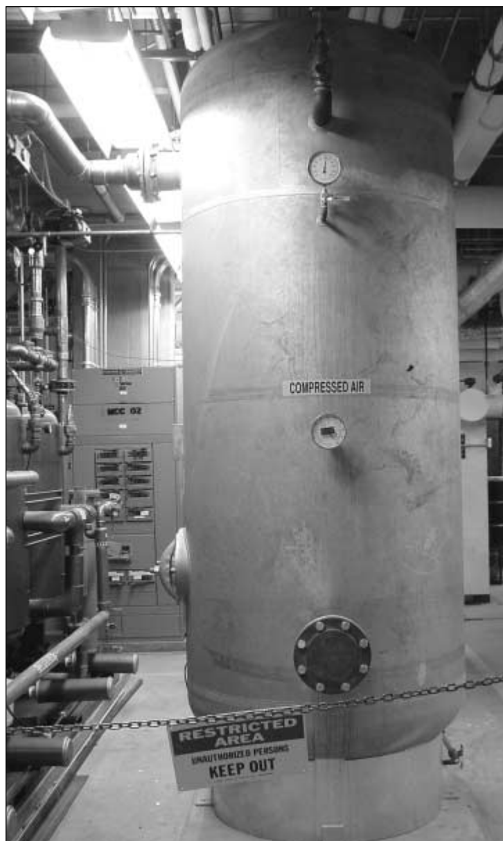
FIGURE 2.15 100 psi compressed air tank.
