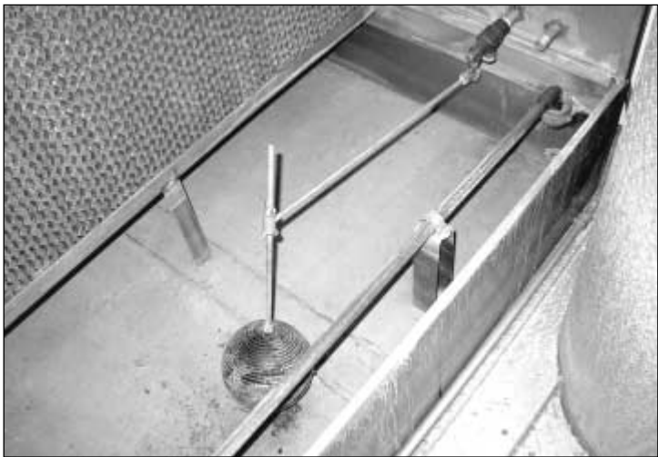
FIGURE 17.9 Swamp cooler sump refill level float not working (no water in pan).
