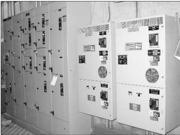
FIGURE 4.13 Motor control center (cabinet on left) and variable frequency drives (two boxes on right).
