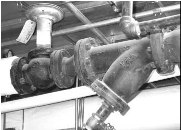
FIGURE 12.4 Steam valve and strainer.
