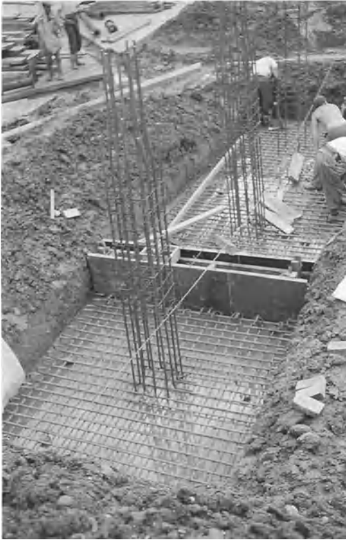
Plate 15a. Column base excavations are always liable to fill with rainwater. A sump should have been excavated beside each to permit dewatering before concreting
