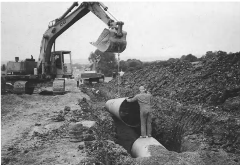
Plate 10b. It is almost universal to use the hydraulic excavator also as a crane
