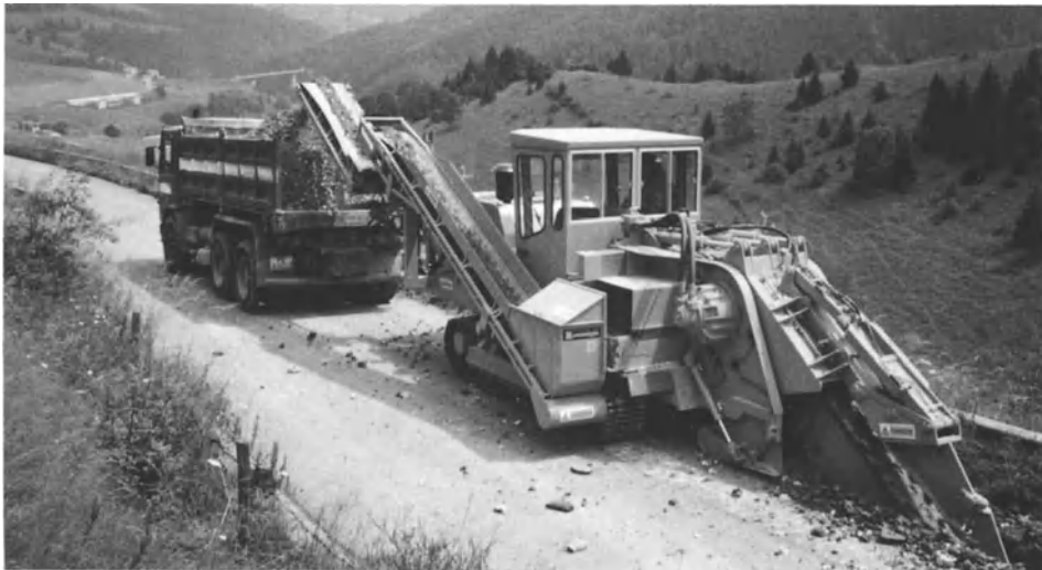
Plate 9b. A Mastenbroek 17/17 trenching machine with variable-offset heavy-duty cutting chain for trenches up to 0.6 m wide by 1.8 m depth. Larger machines are made. J. Mastenbroek & Co. Ltd, Boston, UK
