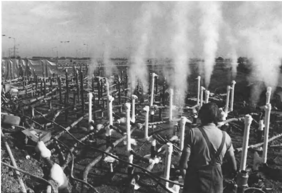
Plate 1b. Ground freezing to permit tunnelling through difficult ground subject to artesian water. Iver treatment works, Three Valleys Water Co., 1984
