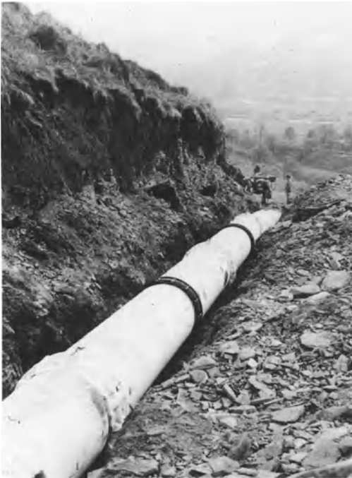
Plate 6a. A problem for the designer under the Construction (Design and Management) Regulations 1994 who has to pay 'adequate regard to the need to avoid foreseeable risks' (see pp. 78–9). The designer may decide a stable berm must be cut into the hillside before the pipe trench is excavated
