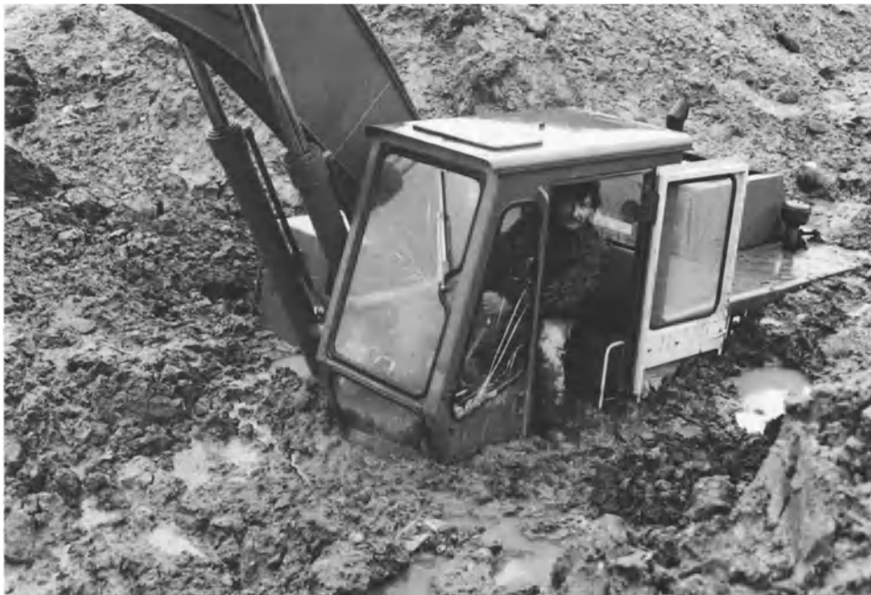
Plate 5b. It can be easier to get out of this sort of trouble than to decide whether the conditions could not reasonably have been foreseen by an experienced contractor' under Clause 12 of the ICE Conditions
