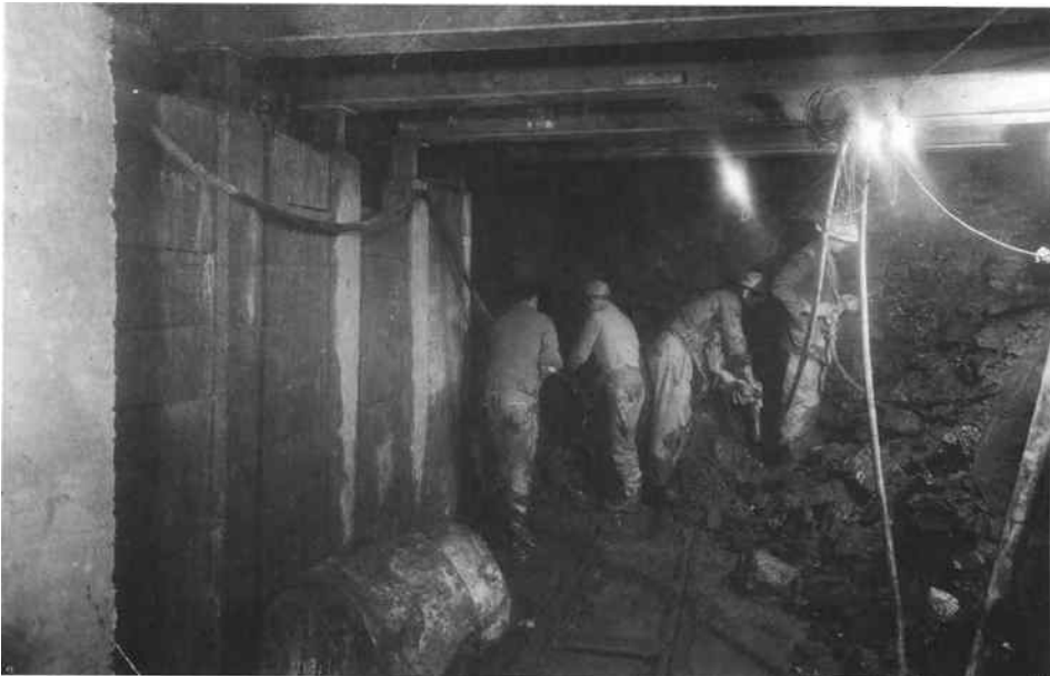
Plate 2b. Tunnel excavation by hand may still be necessary in uncompacted materials requiring instant support. Corrugated steel bars are driven forward over a joist, wedged to slant upwards, so holding the roof material and permitting the next joist to be placed
