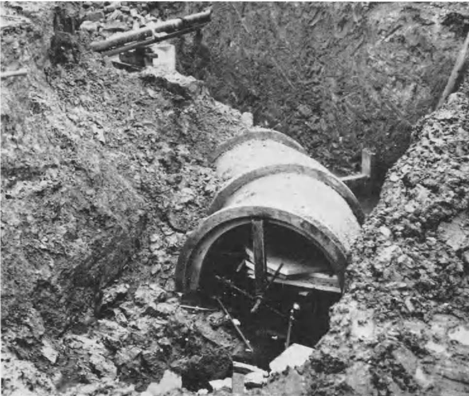
Plate 8b. Presumably somebody thought this trench was stable – and was proved wrong
