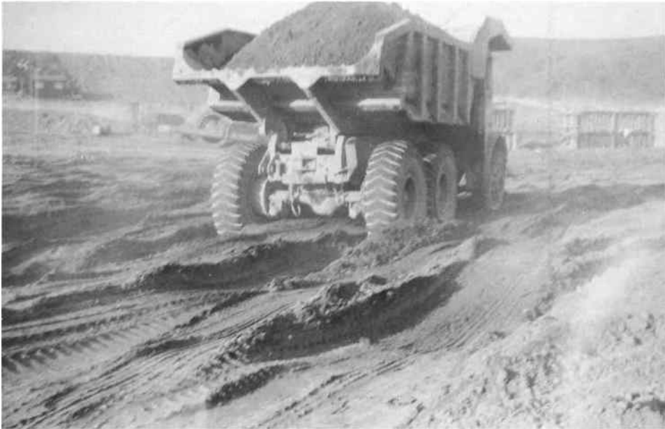
Plate 5a. A badly rutted formation, probably due to excessive moisture content of the fill
