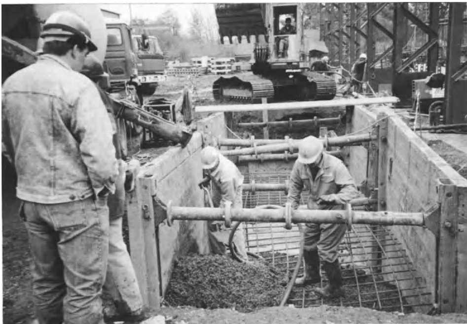
Plate 12b. On any job not properly supervised the strangest things can happen. It looks as if someone forgot the reinforcement until after the first placement of concrete. A resident engineer would stop the work and require it to be redone properly
