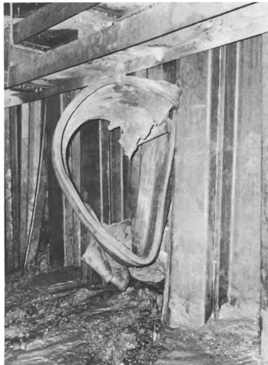
Plate 6b. Steel piling sometimes does not go where the civil engineer thinks it has – especially when he was not aware the ground contained boulders or other obstructions
