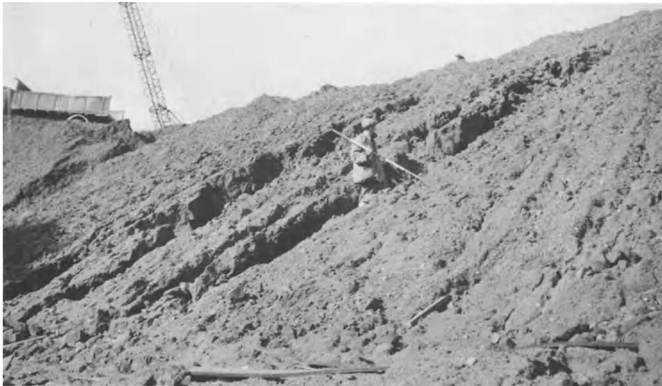
Plate 7b. Erosion of a newly placed embankment by rainfall runoff from the formation above. This is likely to be a contractor's risk, as it is 'a condition due to weather conditions' under ICE Conditions Clause 12
