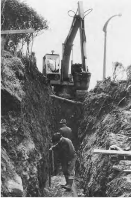
Plate 8a. Accidents can only be prevented by always taking the proper precautions. The trench sides should have been supported, because no one could be certain they would stand unsupported
