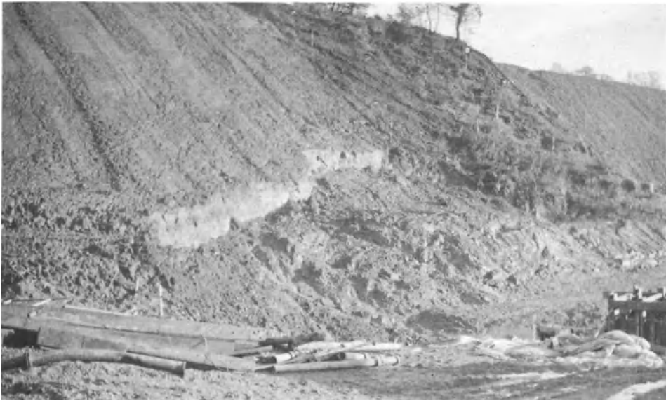
Plate 7a. An unexpected hillside slip in shale. The question is whether it is sensible to place such risks on the contractor
