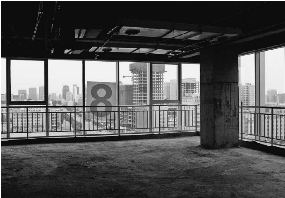
Figure 1.5 Unfinished office complex, Ordos, Inner Mongolia, China
