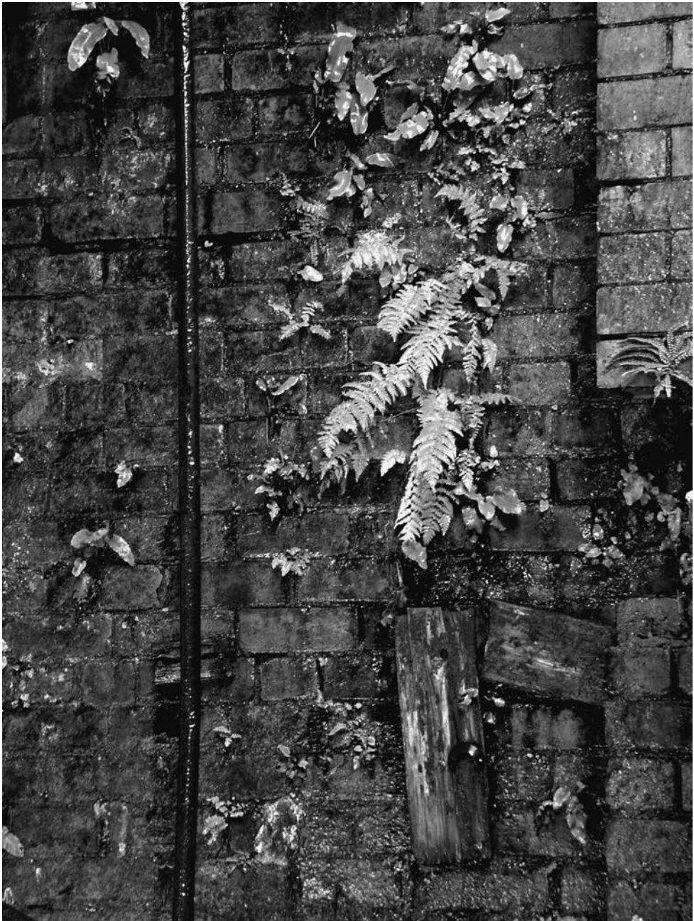
Figure 23.4 Distressed wall, industrial estate, Manchester
