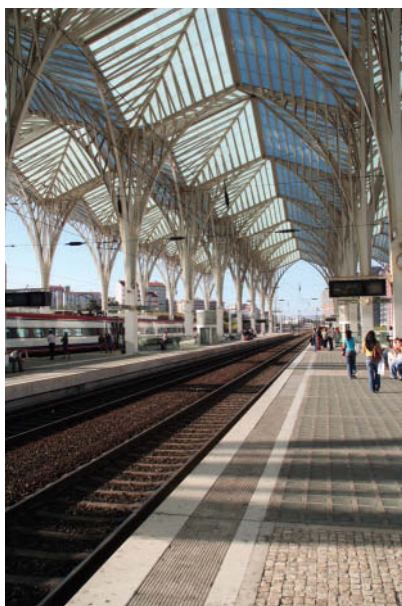
An interesting array of trusses at the Lisbon Oriente Station in Portugal.
