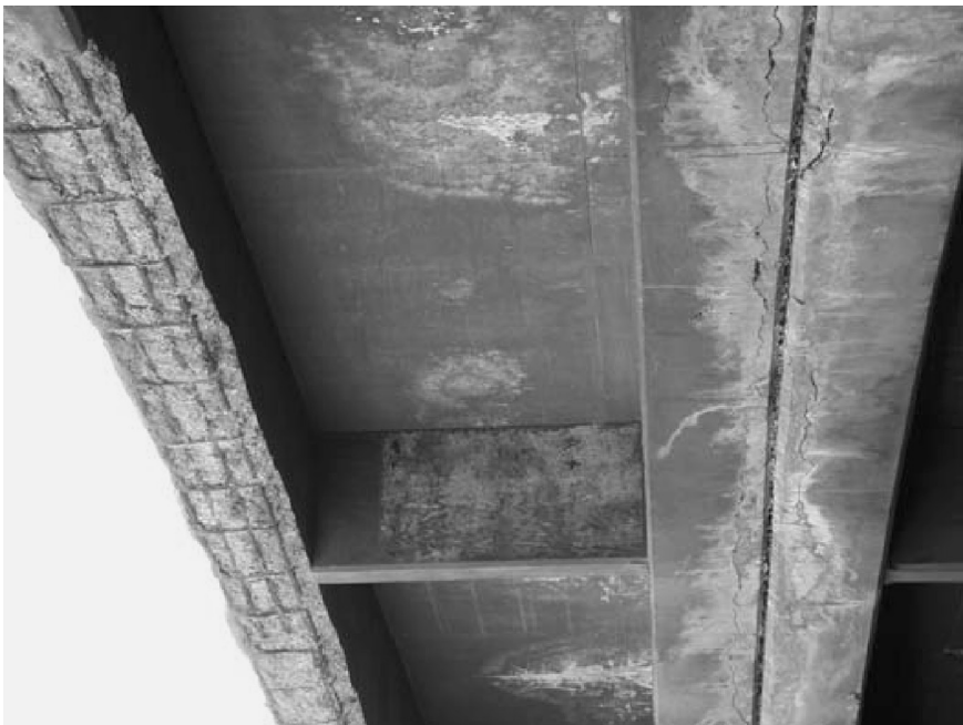
Figure 4.7 Example of steel corrosion.
