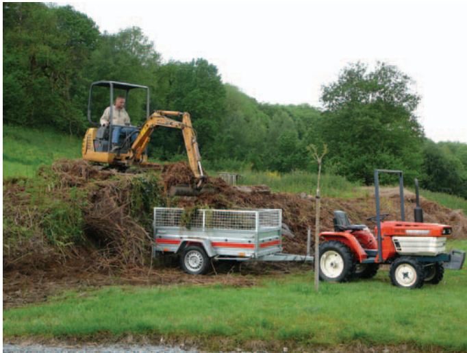
Figure 1.8 Mechanical hazards mobile plant.
