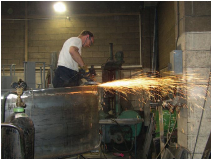
Figure 8.2 Poor working environment.
