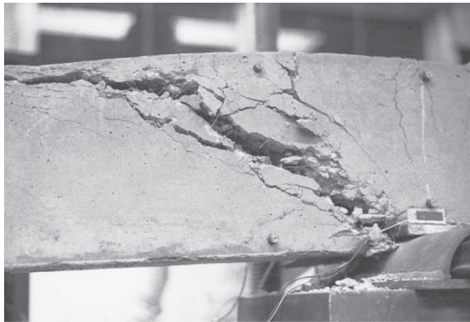
Shear failure near a middle support.
