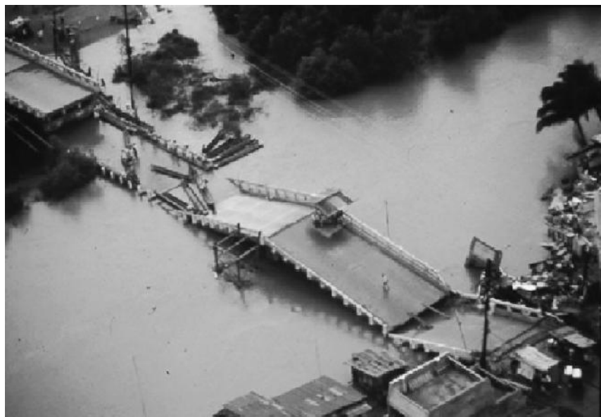
5.7 Infrastructure response to liquefaction: collapse of bridge deck due to liquefaction-induced lateral spreading of embankments and reduced lateral support to bridge piers following the Luzon, Philippines, earthquake of July 1990 (courtesy EEFIT, UK).
