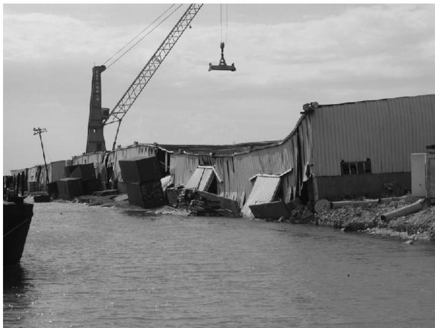
5.9 Damage to port structures and warehouses due to liquefaction-induced lateral spreading following the Haiti earthquake of January 2010 (courtesy EEFIT, UK).
