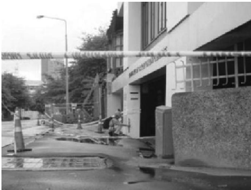
5.10 Damage to foundations in Christchurch, New Zealand, following the earthquakes of 2010 and 2011 showing liquefaction-induced settlement of building foundations (courtesy EEFIT, UK).
