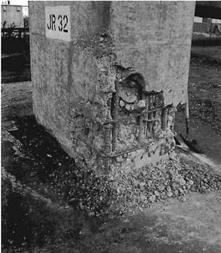
Figure 8.13 Lap splice bond failure during Loma Prieta Earthquake, 1989 (Source: Priestley, M. J. N., Seible, F. and Calvi, G. M., Seismic Design and Retrofit of Bridges , © 1996 and owner. Reproduced with permission of John Wiley & Sons, Inc.).
