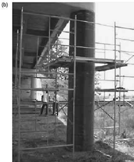
Figure 1.3 Column wrapping with carbon tape, followed by coating of inorganic resin (a) column after cleaning; (b) column wrapped with carbon tape; (c) during final coating application; (d) column after coating (Source: Defazio et al. , 2006).
