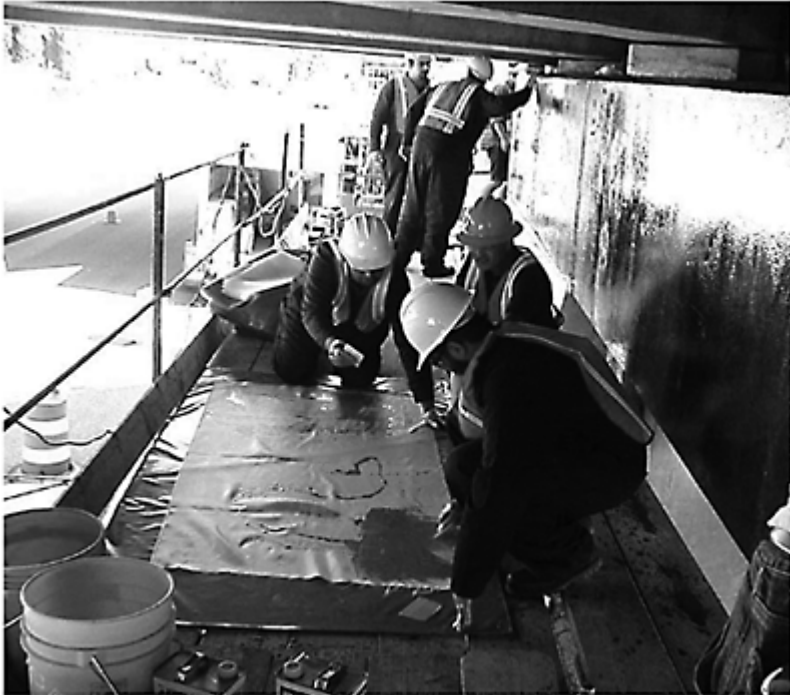
Figure 8.1 Retrofitting with composite material jackets: (a) hand lay-up of fiber-glass with epoxy by the authors; (b) machine winding of carbon fiber and epoxy (Source: XXsys Technologies, Inc., 1997).
