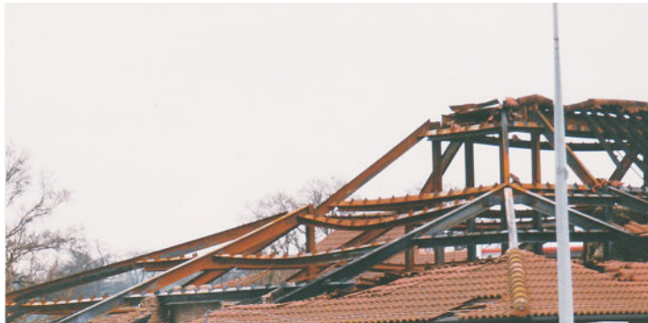
FIGURE 40.1 Steel Frame After a Fire
