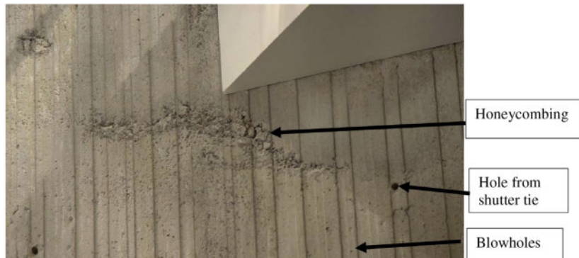
FIGURE 26.4 Defects in Concrete Surface
