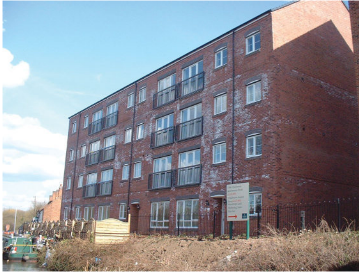
FIGURE 34.4 Severe Efflorescence on New Brickwork
