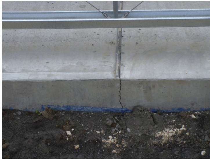
FIGURE 23.6 Crack Caused by Crack Inducer
