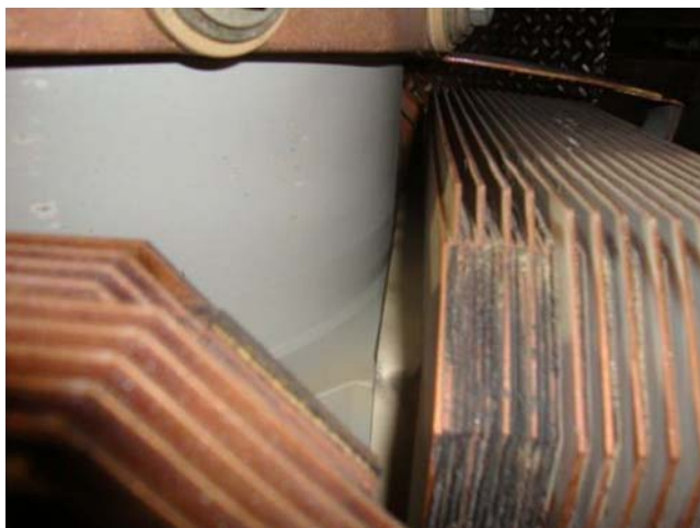
Figure 10.4 Contamination of a strip-on-edge field winding pole.
