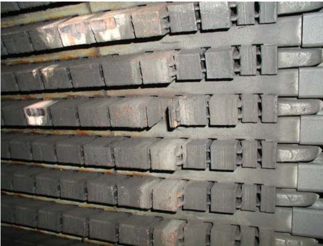
Figure 13.11 Core damage from a loose bolt.
