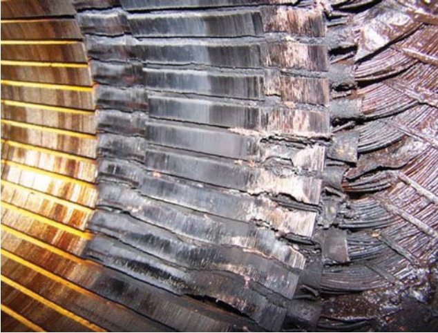
Figure 13.10 Stator rub on bore from bearing failure.
