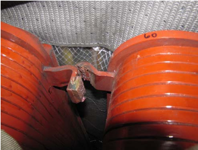
Figure 10.3 Failure of inter-pole connection from thermal cycling.
