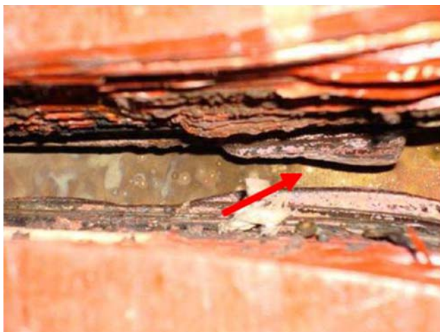
Figure 9.3 Failed pole jumper connection.
