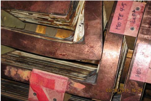
Figure 9.2 End winding copper distortion from thermal cycling.
