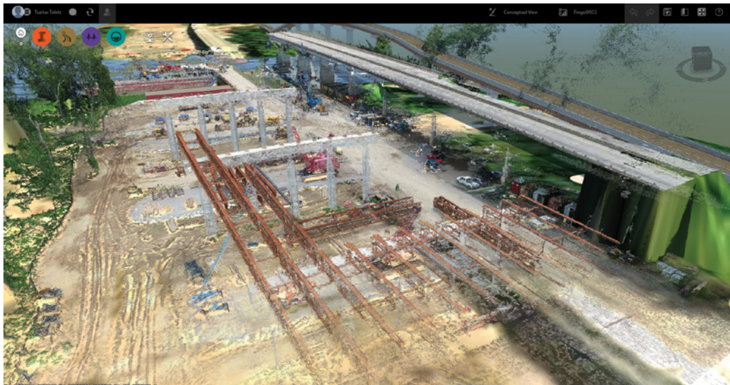
FIGURE 8.5 LiDAR and autonomous drones ease the process of capturing real-time conditions, which can be used for inspection, planning, progress monitoring, and as-built documentation.
